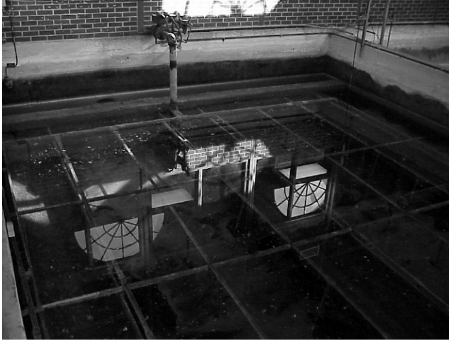
Figure 5-1 Annex (1929) GAC/sand filter.
