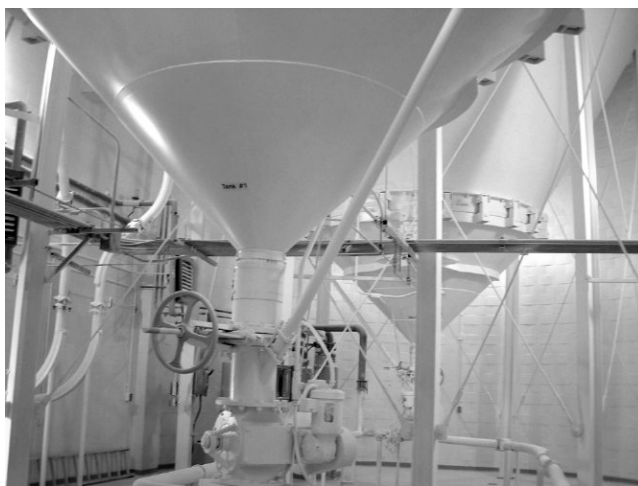
Figure 10-18 Lime storage hoppers.
