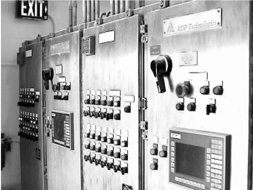
Figure C-10 Control panels indicate each batch phase of lime and water addition, mixing time, temperature, and discharge of slaked lime to continuously-mixed slurry storage tanks.
