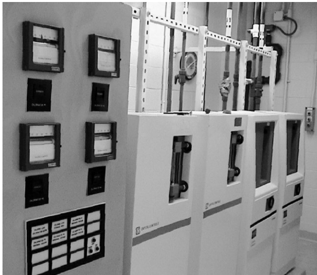
Figure 10-40 Chlorine controls and feeders.
