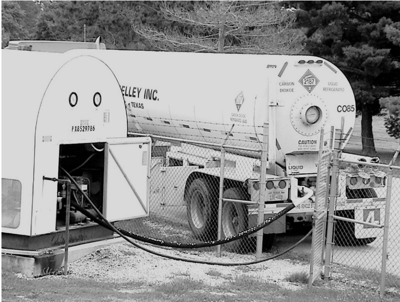
Figure C-14 Carbon dioxide is fed to east and west recarbonation basins to reduce pH of lime-softened water.
