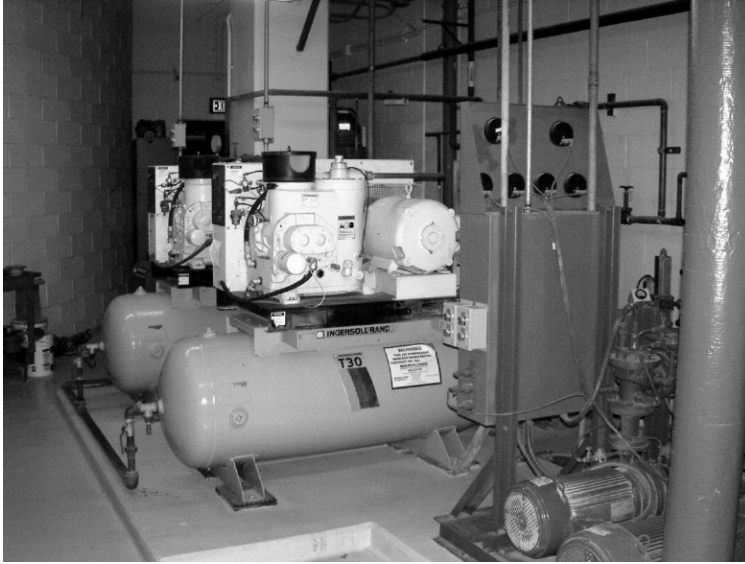
Figure C-8 Compressors, vital to operation of valves, are checked for performance, pressure, unusual sounds.
