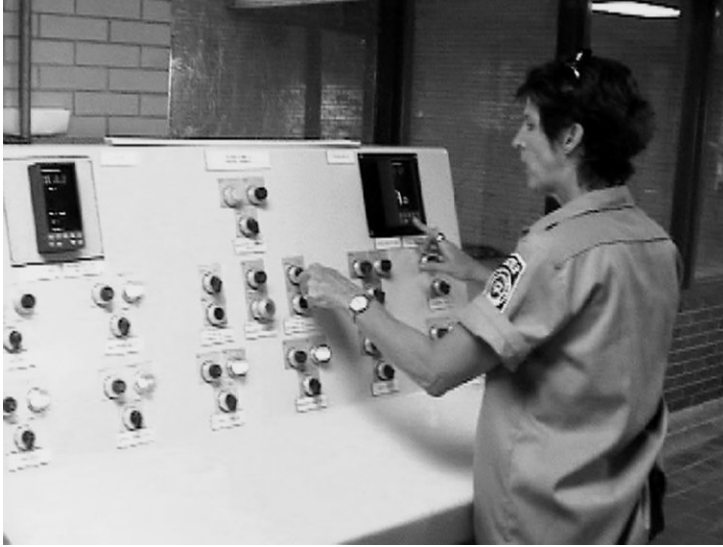
Figure C-16 Filter backwash requires filter draining, opening backwash valves, activating pump #1 for initial bed expansion, then pump #2 for further expansion.
