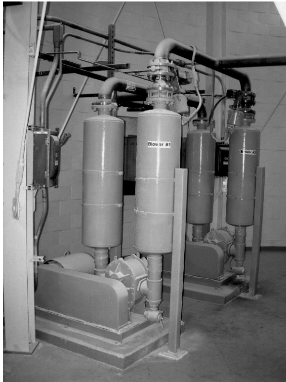
Figure C-26 Blowers are used to transfer powdered lime from bulk storage to a feed hopper atop slakers.
