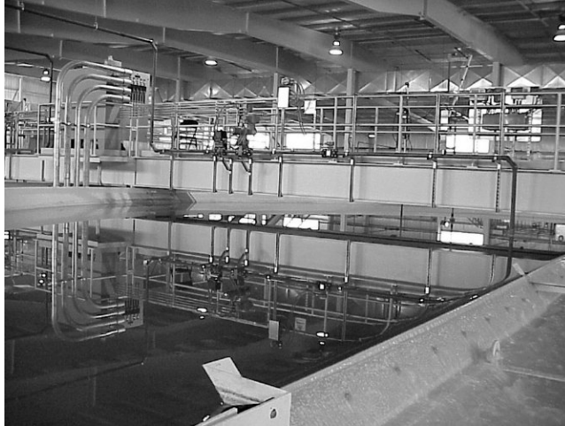
Figure 10-31 Enclosed building houses four ClariCones.
