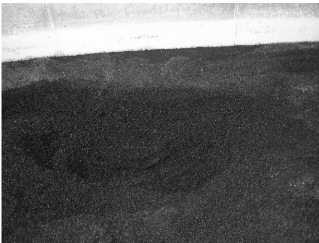
Figure 5-2 Granular activated carbon filter cap.
