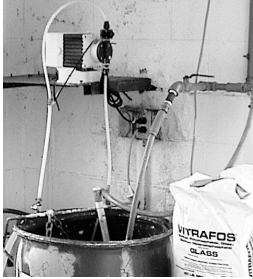
Figure 10-37 Hexametaphosphate is fed to effluent of recarbonation basin.
