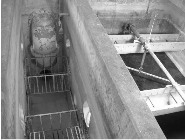
Figure 5-11 Main Building filter wash water gullet.
