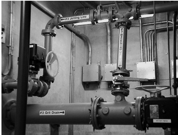
Figure C-36 Piping for jetting and grit removal.
