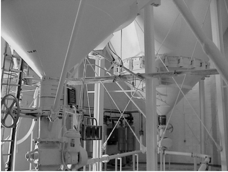
Figure C-25 Lime storage hoppers.
