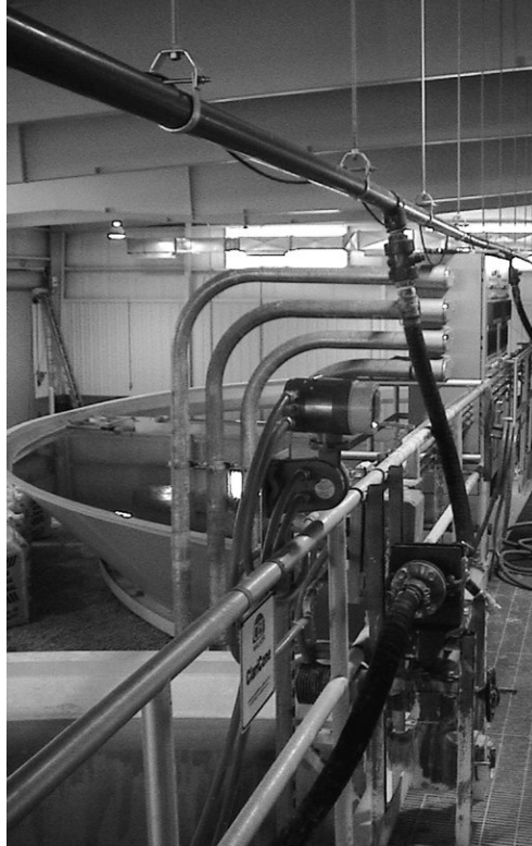
Figure 7-1 Modified lime slurry feed system (flexible hoses from overhead recirculating slurry line).
