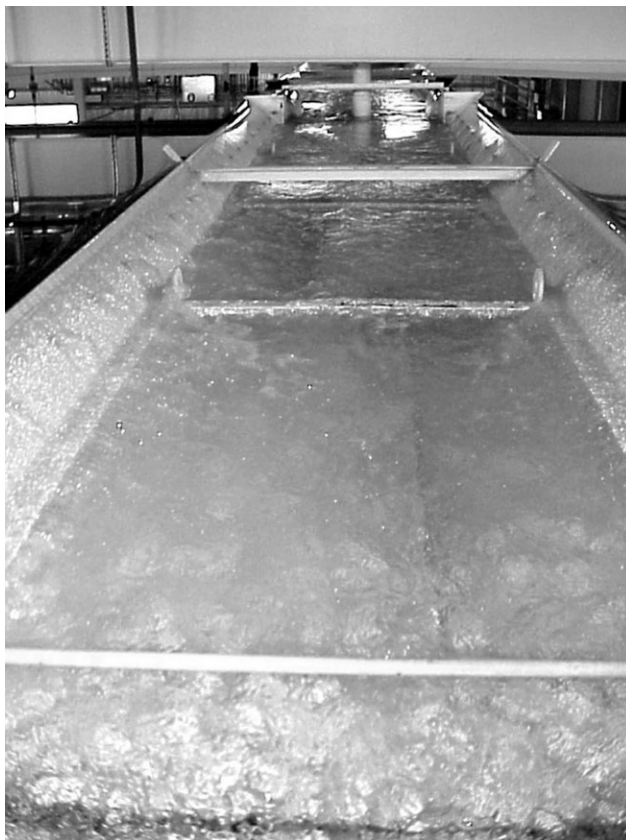
Figure 7-8 ClariCone effluent trough.
