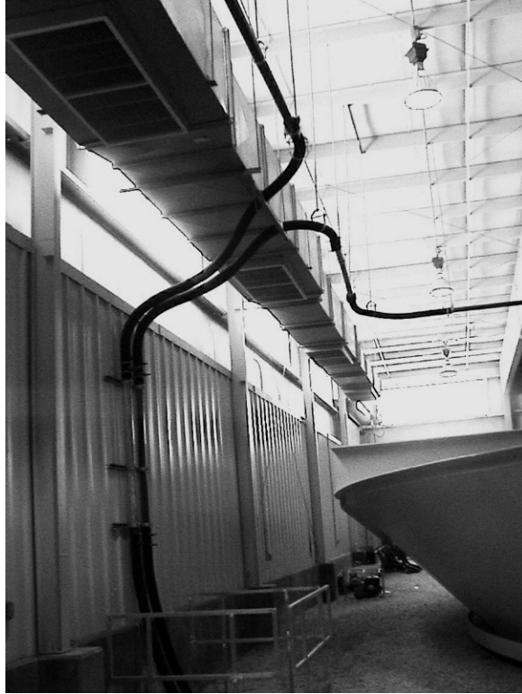
Figure C-30 Lime recirculation system is hung from the ceiling.
