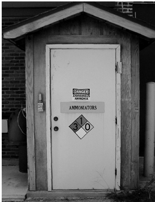
Figure 10-42 Ammonia gas feed outbuilding.
