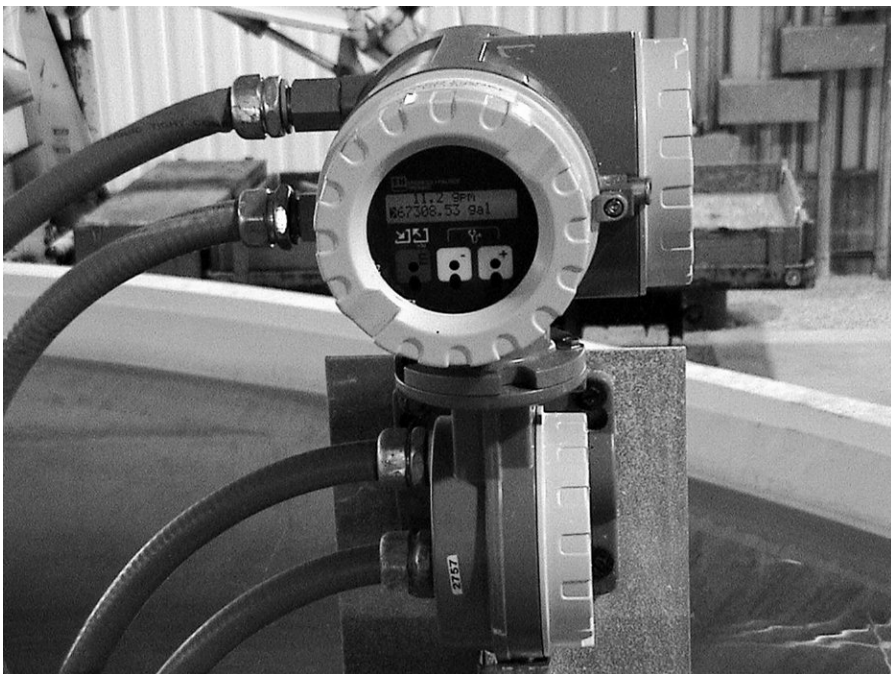
Figure C-33 Flow meter and controller.
