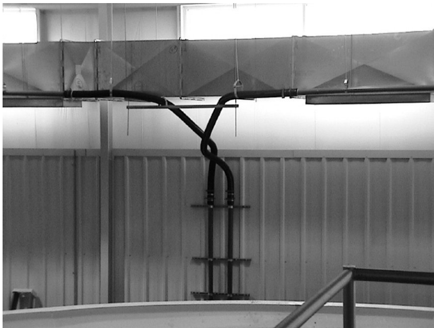
Figure 10-27 Lime slurry piping to softeners.
