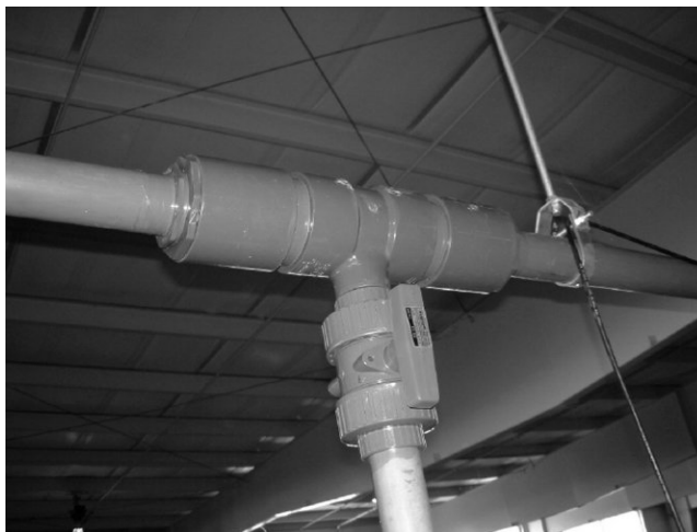
Figure 10-29 Vertical lime slurry PVC distribution pipe.
