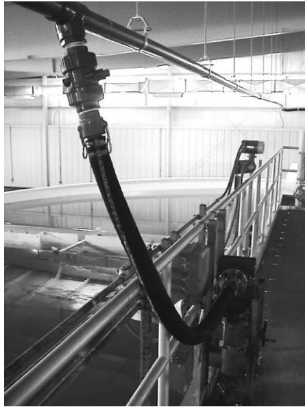
Figure 8-9 Lime slurry pipe loop.
