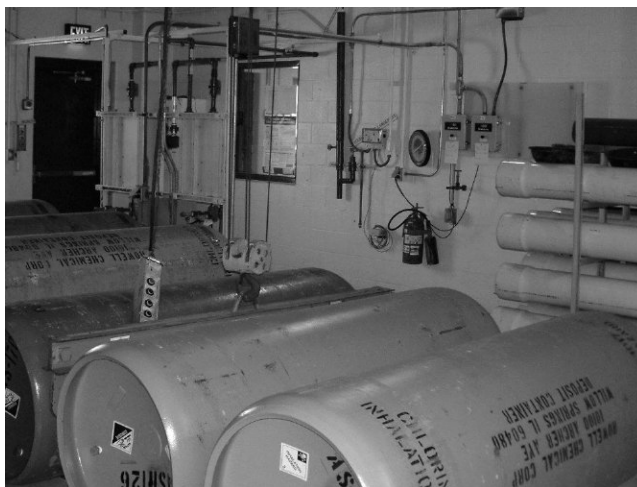
Figure 10-38 Chlorine cylinder storage and feed controls, alarms.
