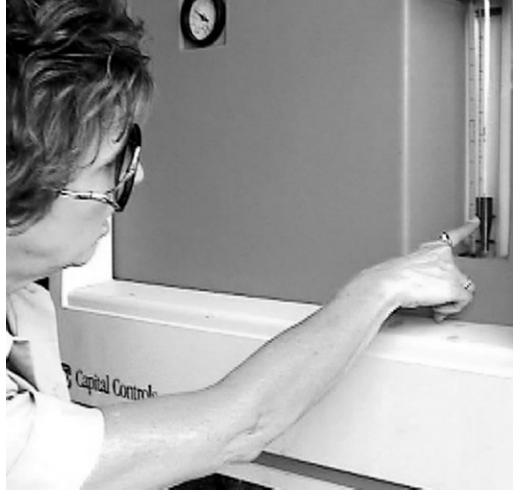
Figure C-6 The chlorine gas feed system is checked for leaks, odors, icing, and a satisfactory feed rate that will ensure a combined chlorine, finished water residual. Subsequently, one part of ammonia is fed per 3.5 parts of chlorine.
