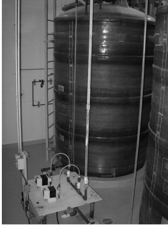
Figure 10-32 Hydrofluosilicic acid bulk storage tank and feed pumps.
