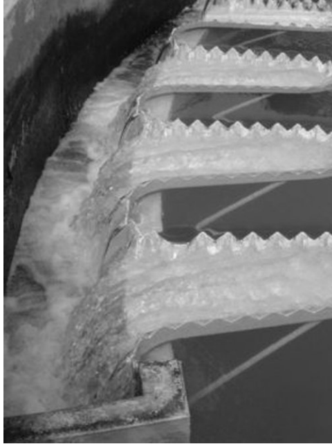
Figure 4-3 Calcium carbonate on recarbonation basin effluent launders.
