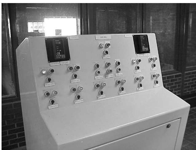
Figure 5-10 Main Building filter control console.
