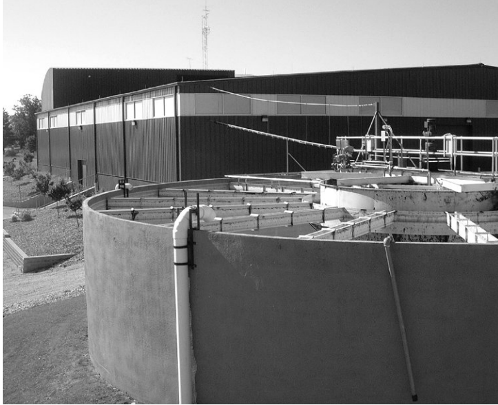
Figure 1-3 Lime softening units: external and housed.
