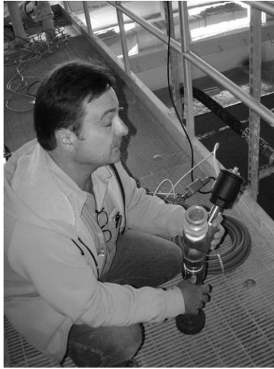
Figure 7-12 Grit removal apparatus.
