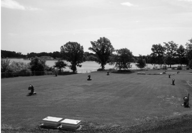
Figure 10-15 Underground finished water storage reservoir.
