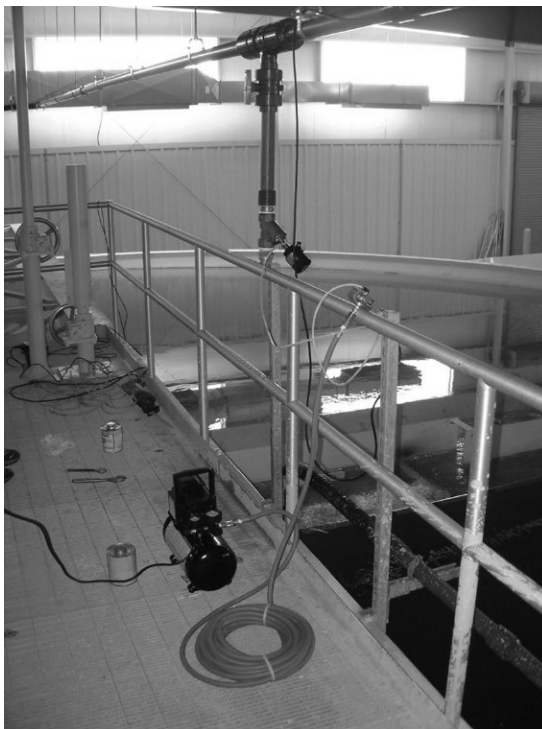
Figure 7-17 Air compressor and hose.
