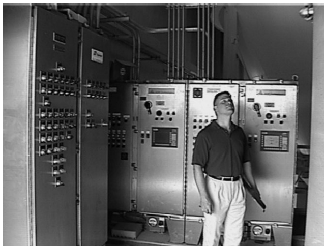
Figure 10-23 Control panel for slakers.
