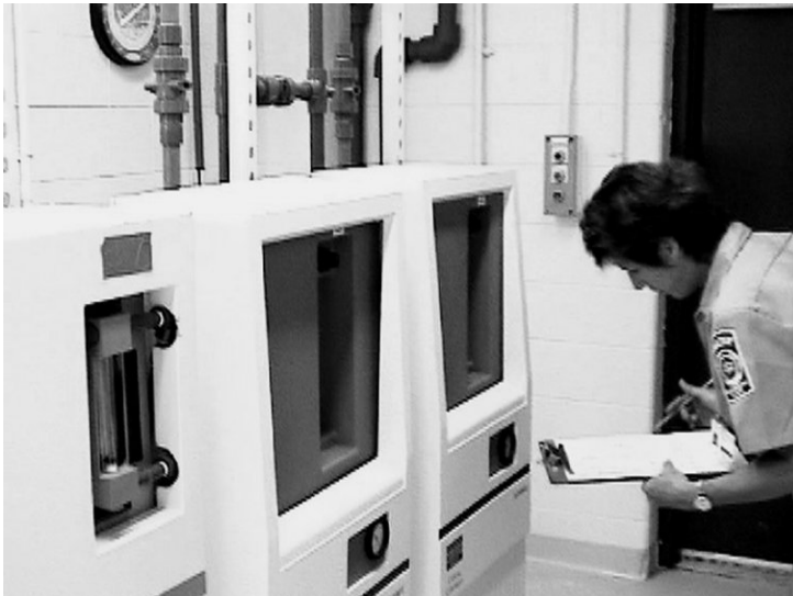
Figure C-13 Rotameter gas feed rates must be adjusted whenever plant flow rates are changed to match system demand.
