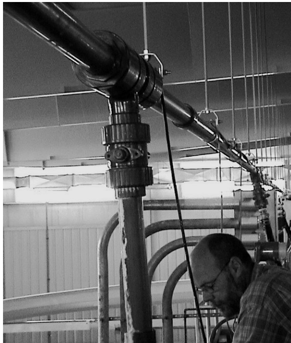
Figure C-31 Valved PVC pipes deliver lime slurry to each softening unit.
