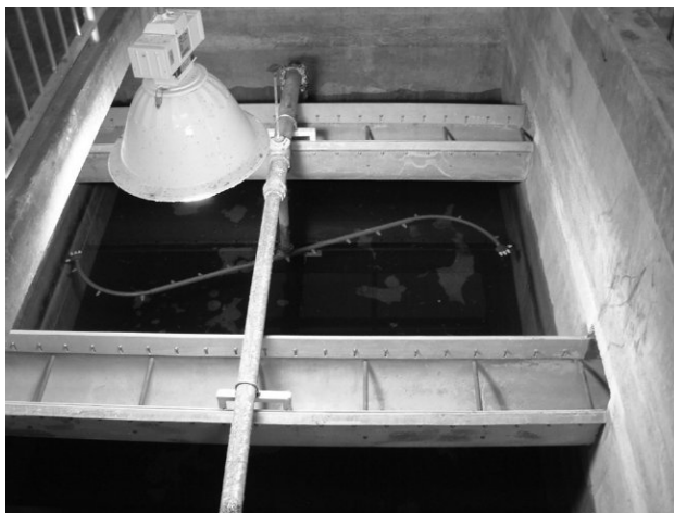
Figure 5-4 Main Building GAC/sand filter.
