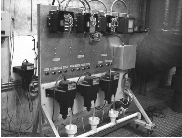
Figure 10-46 Panel designed to monitor both acidified and unacidified filtered water turbidity.
