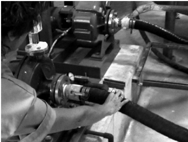
Figure C-11 Slurry storage tanks, flexible hose, couplings, and lime slurry pumps are checked for leaks and incipient ruptures.
