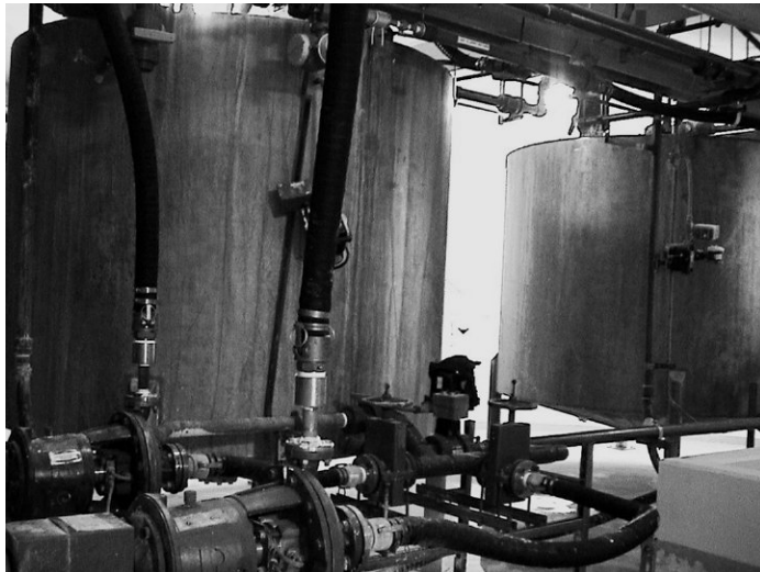
Figure C-28 Slaked lime storage and recirculation system.
