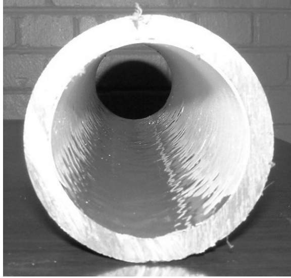
Figure 10-28 Grit-abraded invert of PVC pipe.
