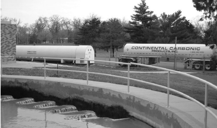
Figure 10-35 Recarbonation basin, carbon dioxide storage tank, and supply tanker truck.
