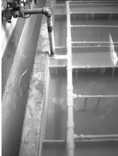
Figure 5-3 Filters in 1929 Annex have fixed surface wash nozzles.
