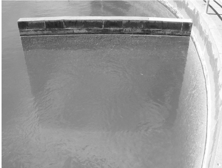
Figure 6-16 Recarbonation basin under normal operating conditions.
