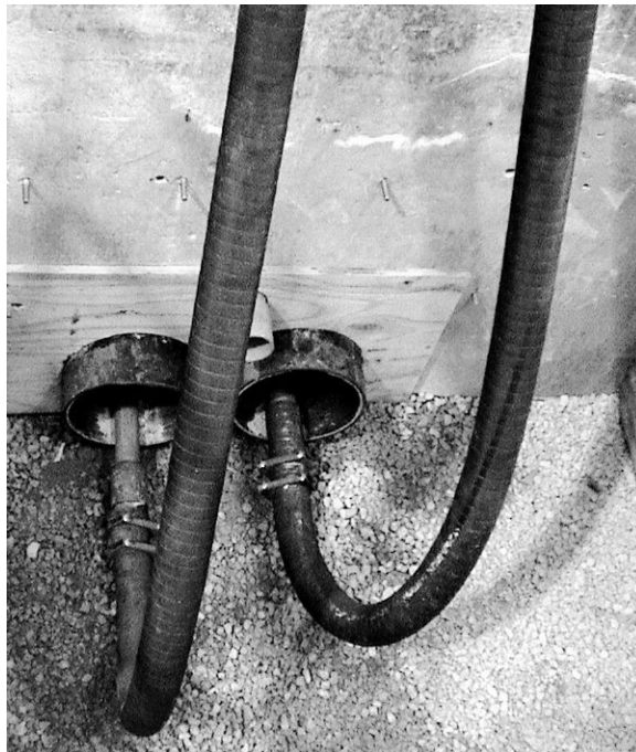
Figure C-29 Lime slurry feed lines entering and leaving softener building.
