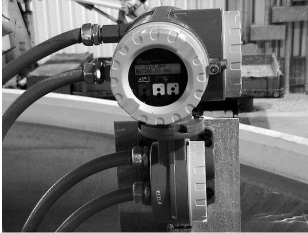
Figure 7-3 Lime slurry flow meter sends rate data to flow controller.
