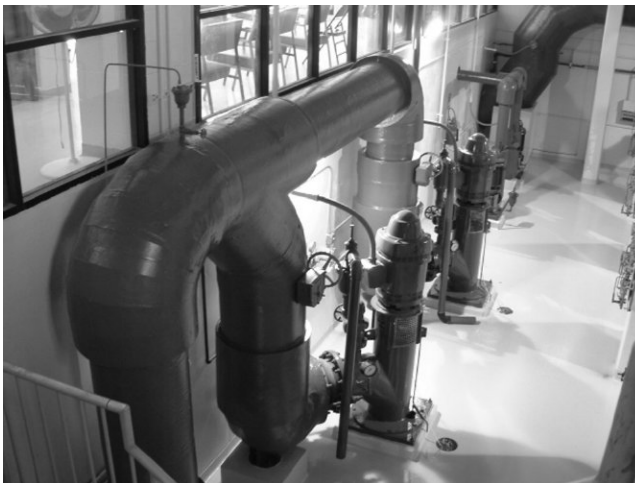
Figure 10-47 High-lift pumps to distribution system.
