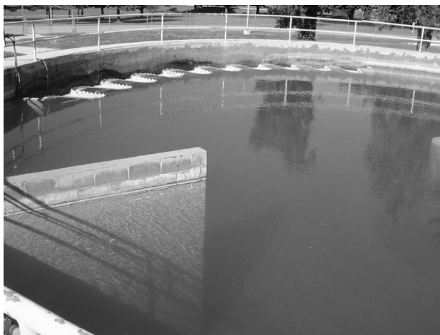
Figure 7-10 Recarbonation basin showing serpentine effluent launders (background) and baffle wall.
