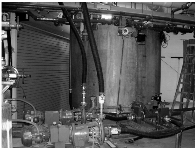
Figure 10-25 Slaked lime slurry storage, mixing, and recirculating pumps.
