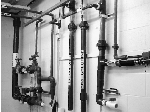
Figure 10-41 Distribution of chlorine solution.
