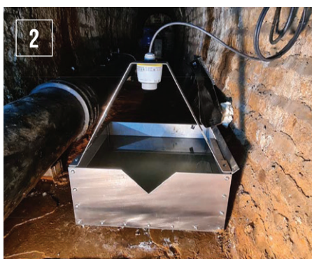
1 Figure 1 – Standard C&RT Telemetry Kiosk
