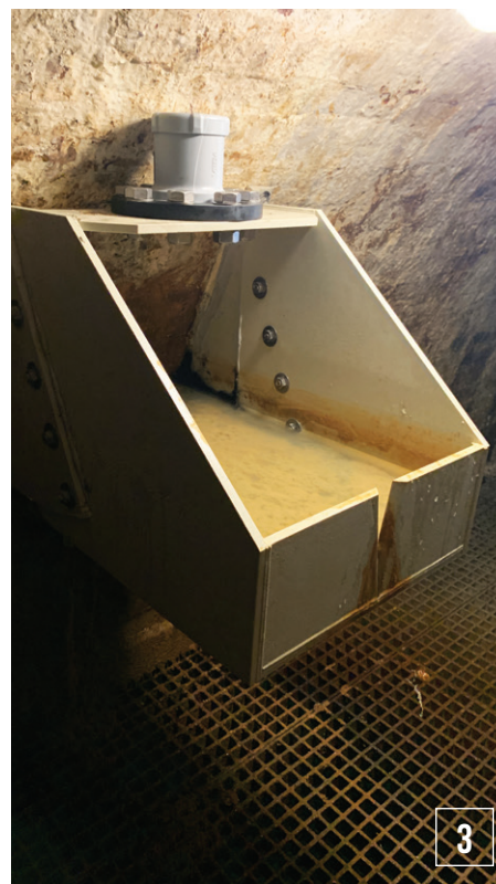
3 Figure 3- VEGAPULS Air 42 on a V-notch flow box
