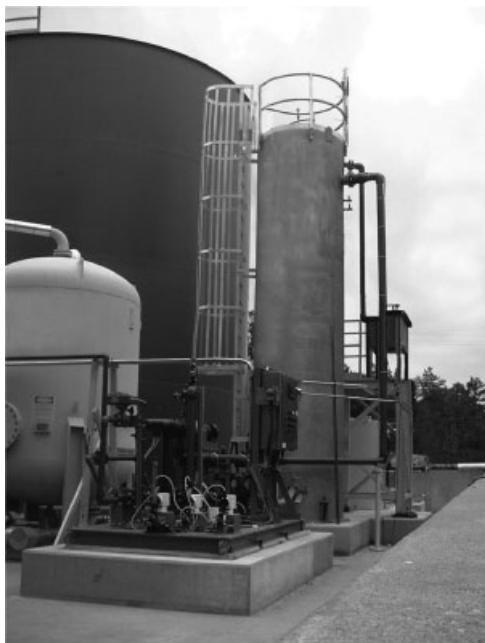
Figure 10.7 Full-scale GAC-FBR system to treat groundwater at LHAAP in Texas, USA [17](permission received).
