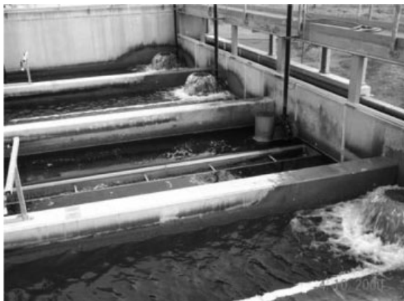
Figure 5.7 Four parallel BAC reactors in the South Caboolture Water Reclamation Plant [23]. (permission received)
