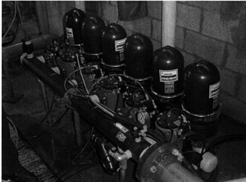
Figure 31 Filters at the Frank Bay plant
