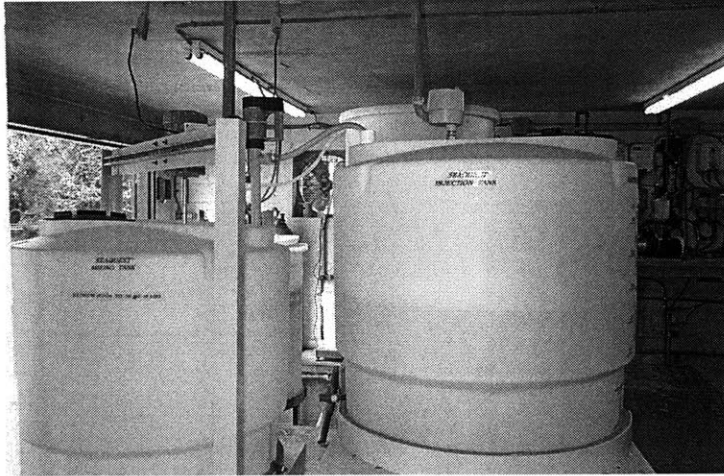
Figure 19 Chlorine storage tanks
