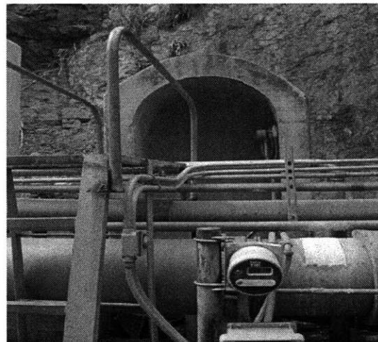
Figure 25b Brine discharge point
