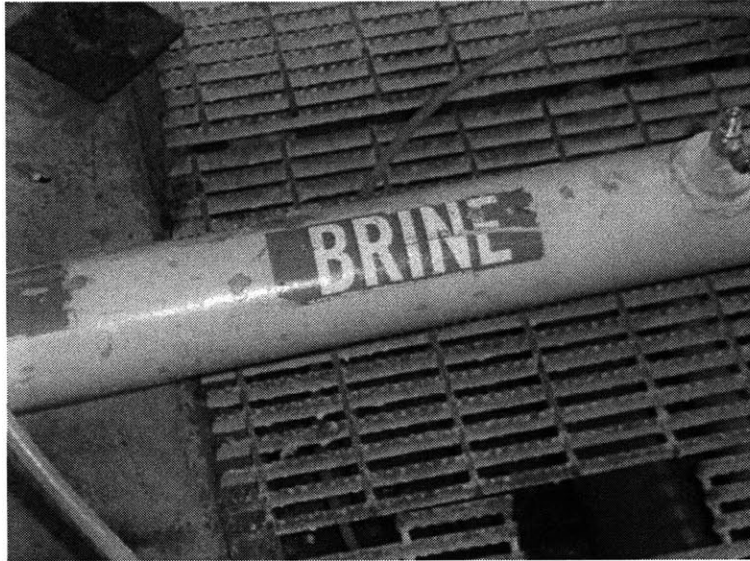
Figure 38 Brine discharge pipe at Frank Bay desalination pipe
