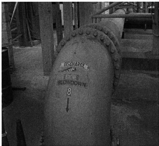
Figure 25a Brine discharge pipe
