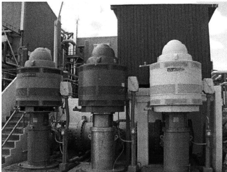
Figure 18 Feedwater intake pumps at the Water and Power Authority Krum Bay Plant
