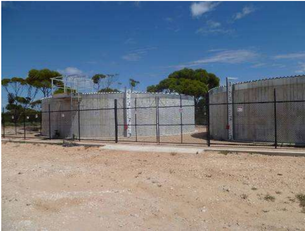
Figure 6–2: Yalata raw water storage tanks
