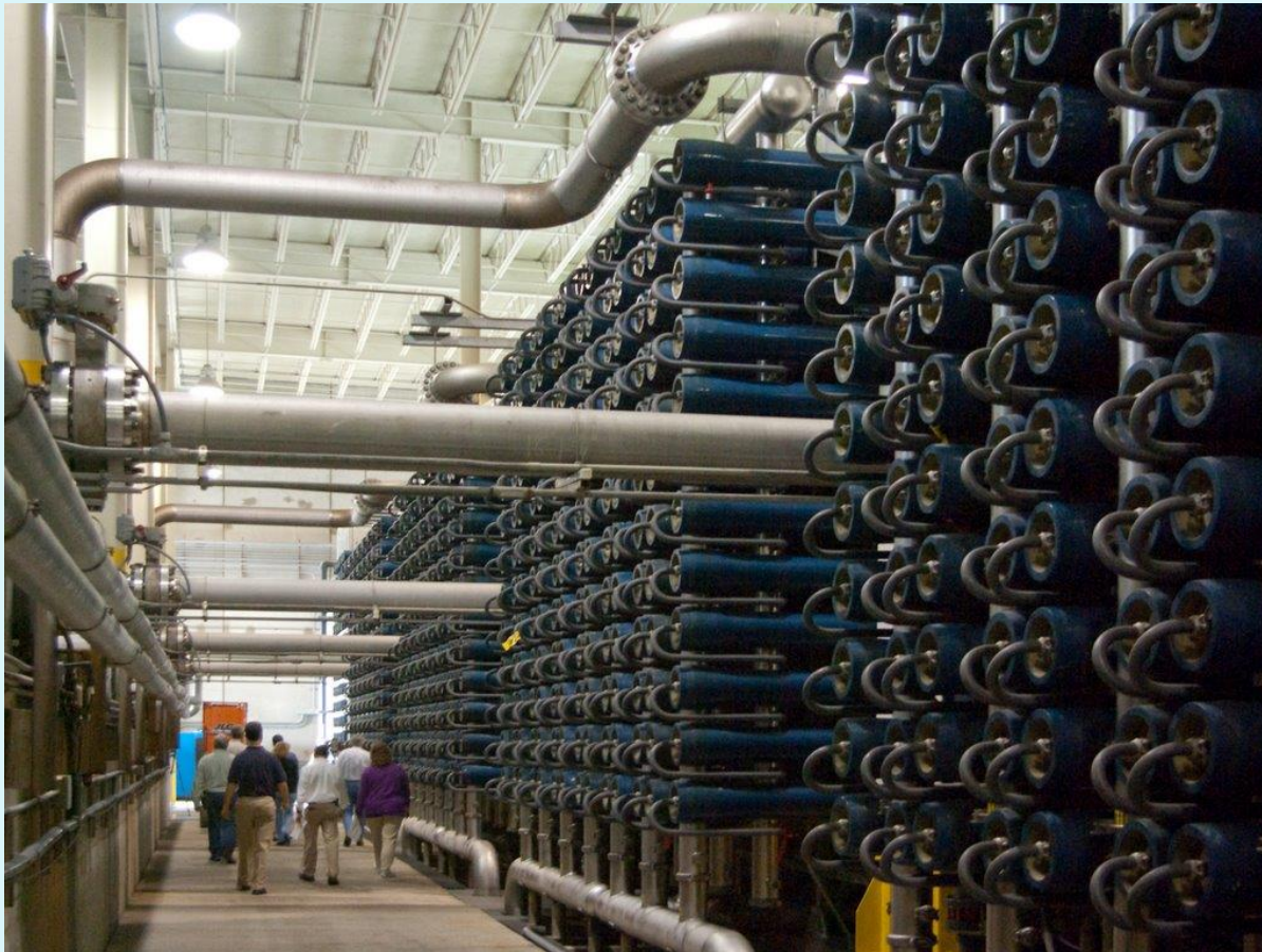
Tampa Bay RO Desalination Plant, Florida, US, 2007
