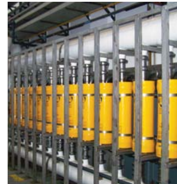
Turbine ERD Retrofit at Empresa Mixta de Aguas de Las Palmas, S.A (EMALSA) Desalination Plant. Facility wins Best Energy Efficiency Project at InfoPower and InfoEnviro's 1 st Annual Energy and Environment Awards in 2012 in Spain.
