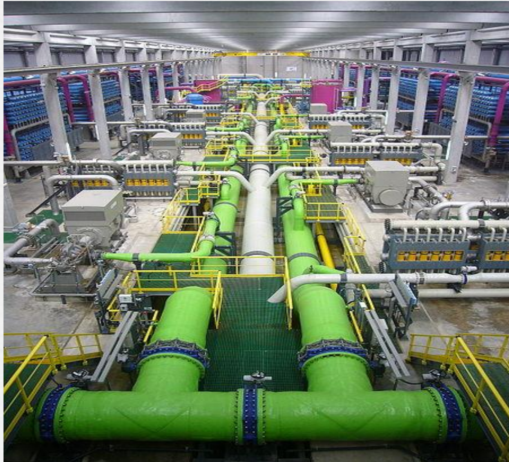
Reverse Osmosis Desalination Plant
