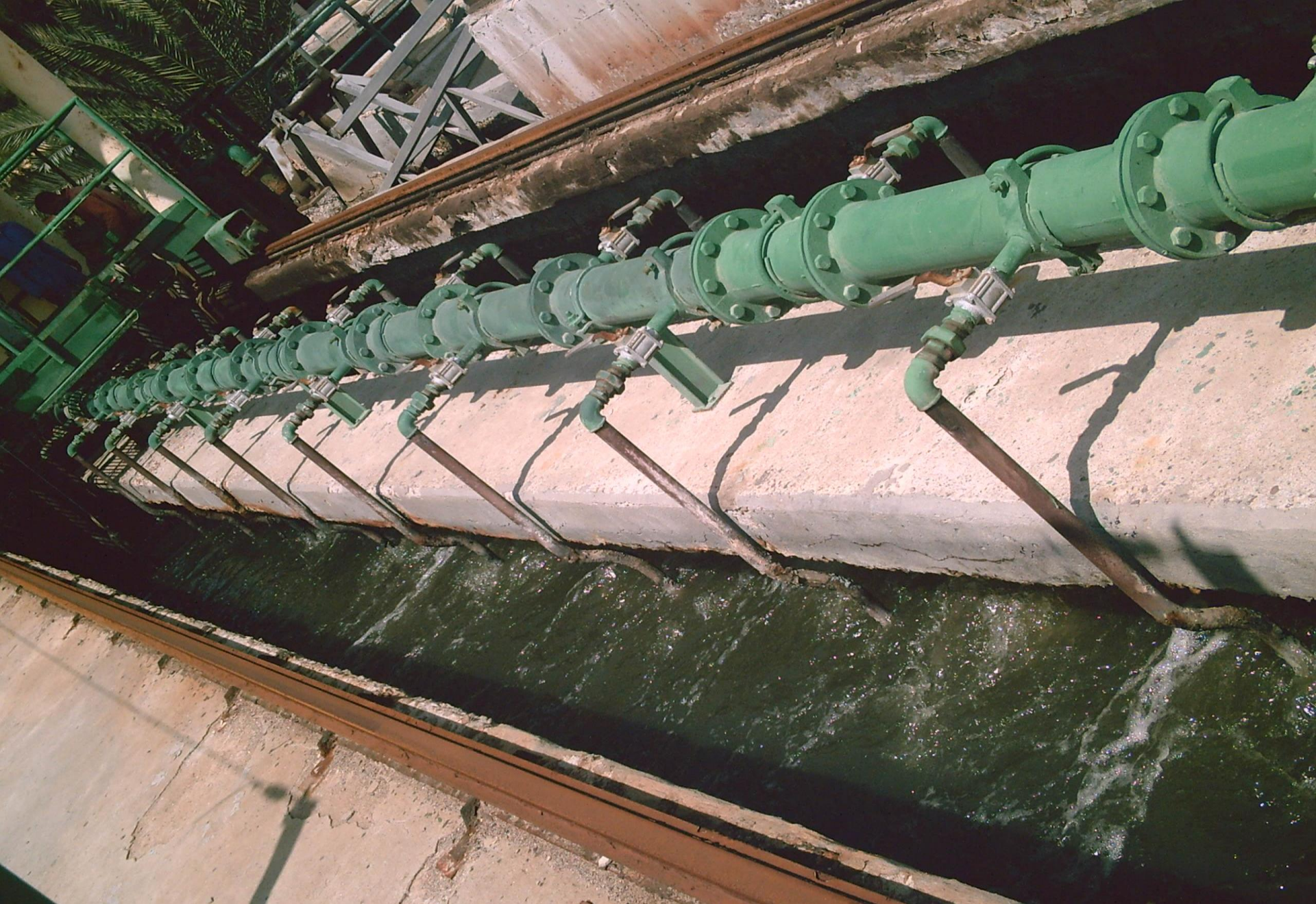
Compressed Air Pipe
