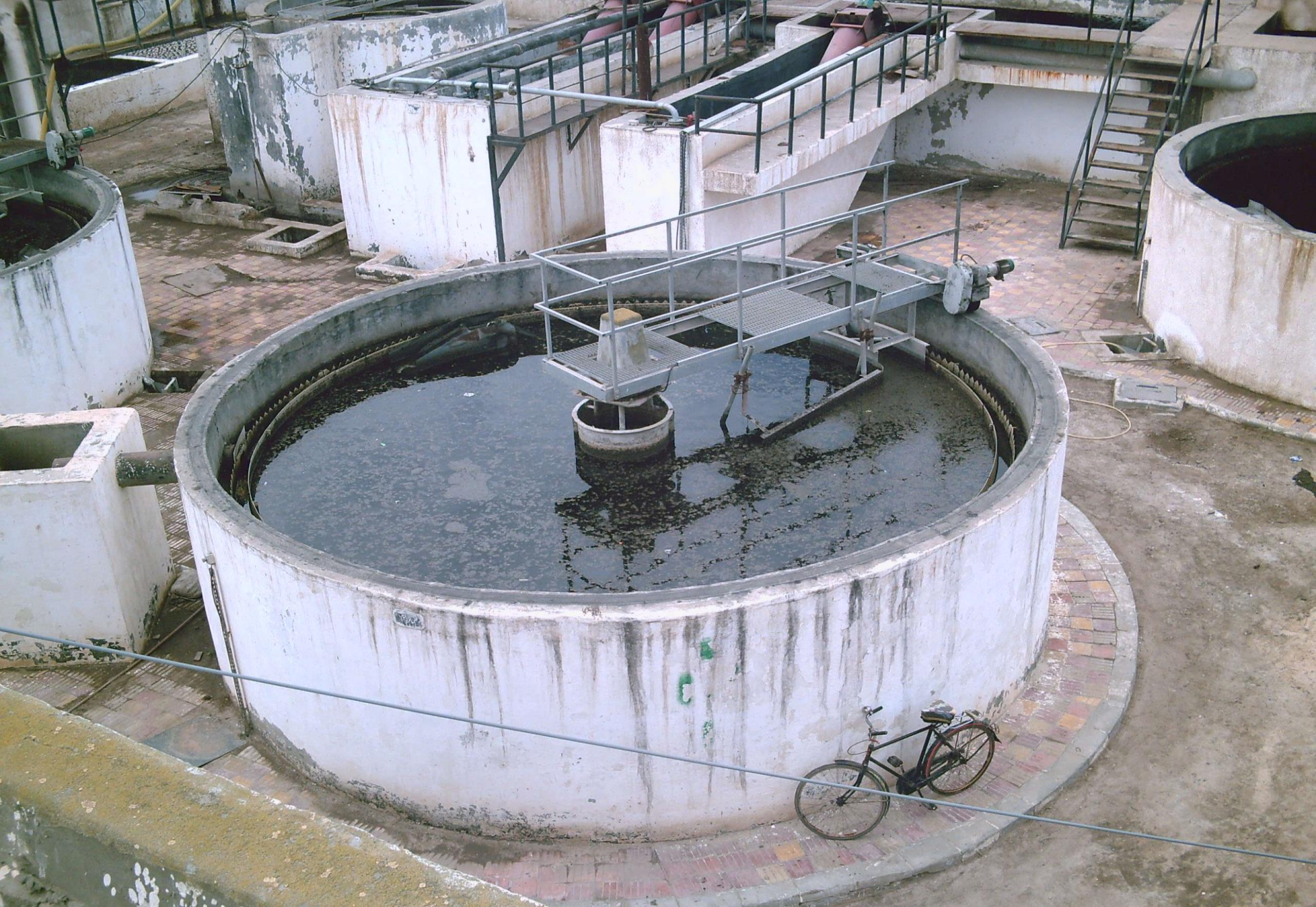
Final Sedimentation Tank
