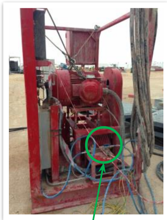
Test Pump Manifold
