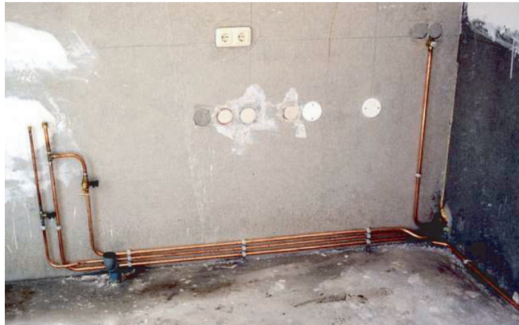
Figure 4.38. Indoor installations made of copper.
