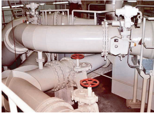
Figure 4.76. Piping in pumping station.
