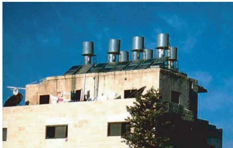
Figure 1.14. Roof tanks in Ramallah, Palestine (Trifunović, Abu-Madi, 1999).
