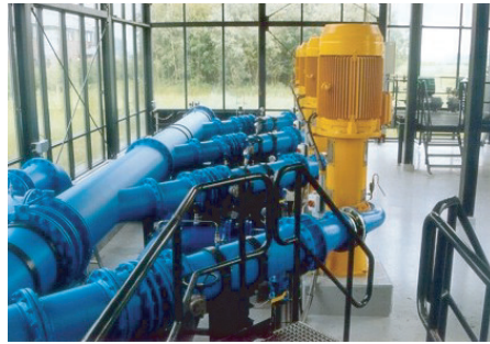
Figure 4.78. Unmanned booster pumping station.
