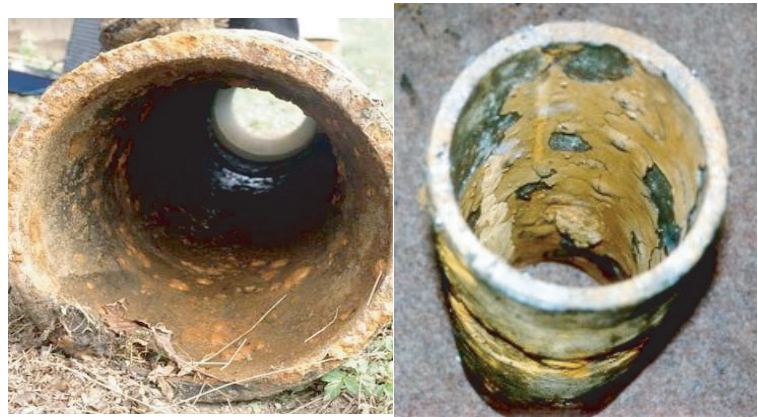
Figure 4.32. Old cast iron pipes.
