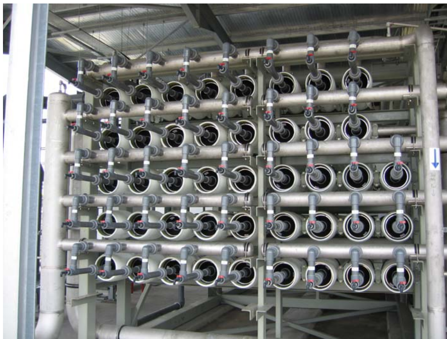
Figure 11. United Envirotech. Reverse osmosis modules
