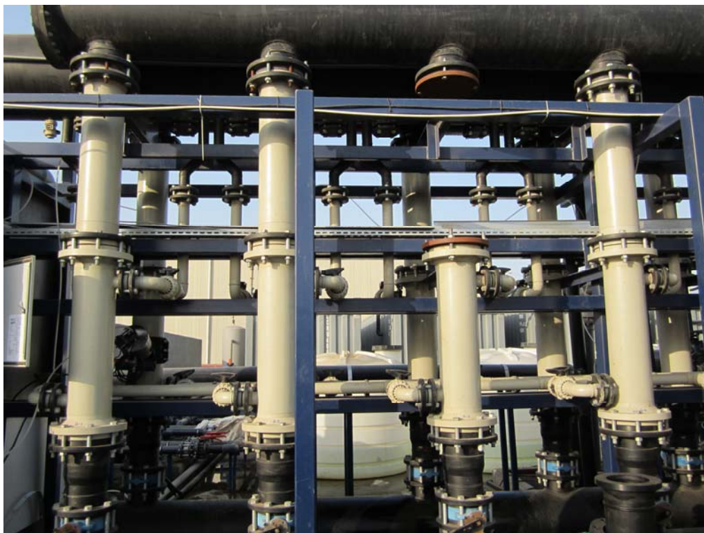
Figure 7. LIQTECH. Ultrafiltration system for a 70 m 3 /h flow. Textile ETP (Egipt).
