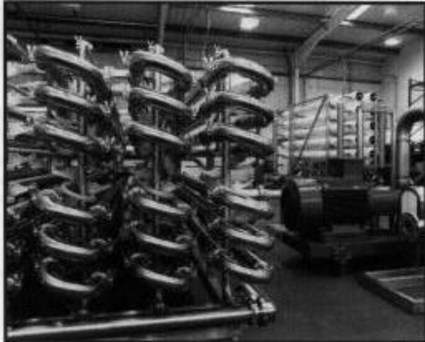
Figure 1. This membrane filtration installation involves two-stage processing of petrochemical plant wastewater. UF unit (left foreground) provides initial separation of particulates and solids, while the spiral membrane reverse-osmosis unit (right background) separates water for re-use and polyol for incineration with the particulate waste.
