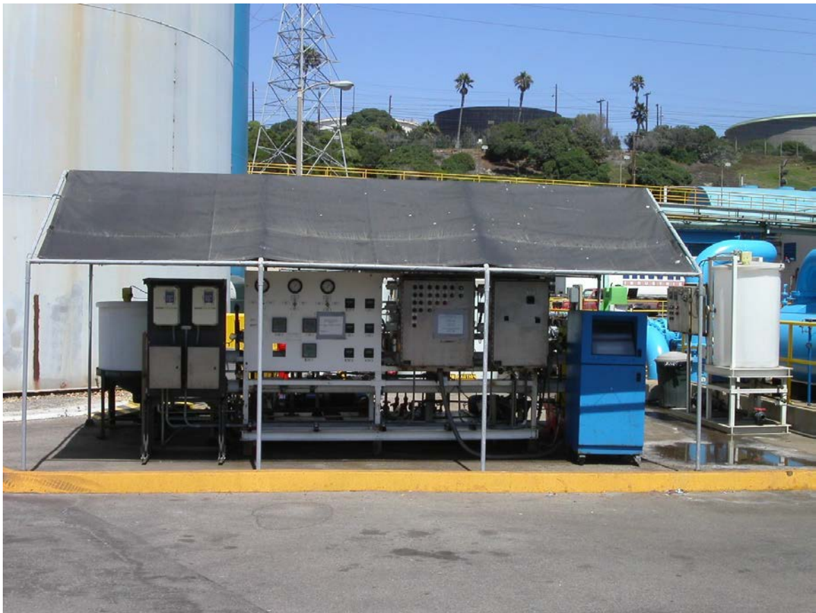
Figure 1.—Pilot test equipment at the El Segundo Powerplant.
