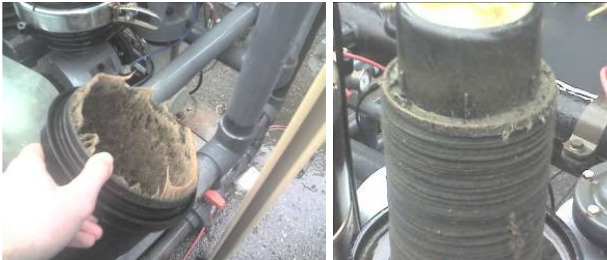
Figure 59.—Biogrowth in Arkal filter housing.
