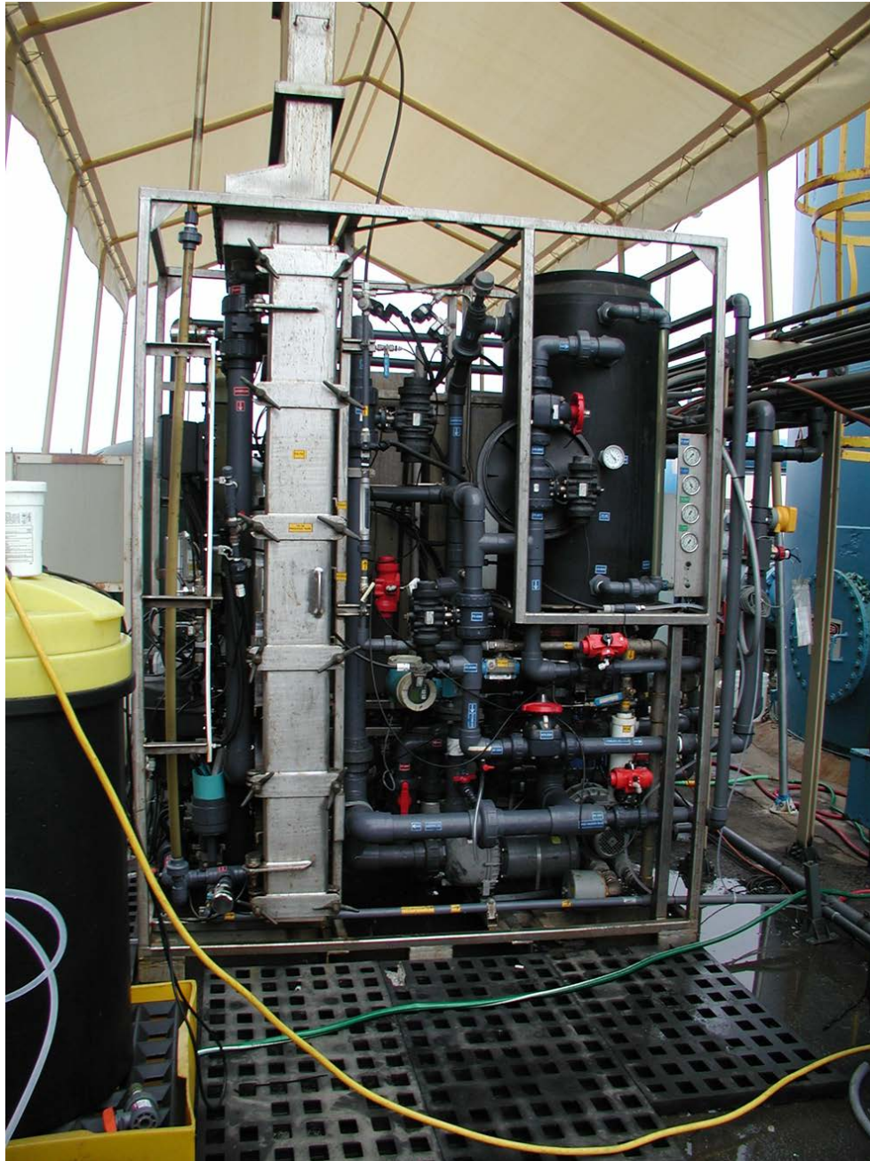
Figure 30.—Zenon ZW1000 ultrafiltration pilot system.
