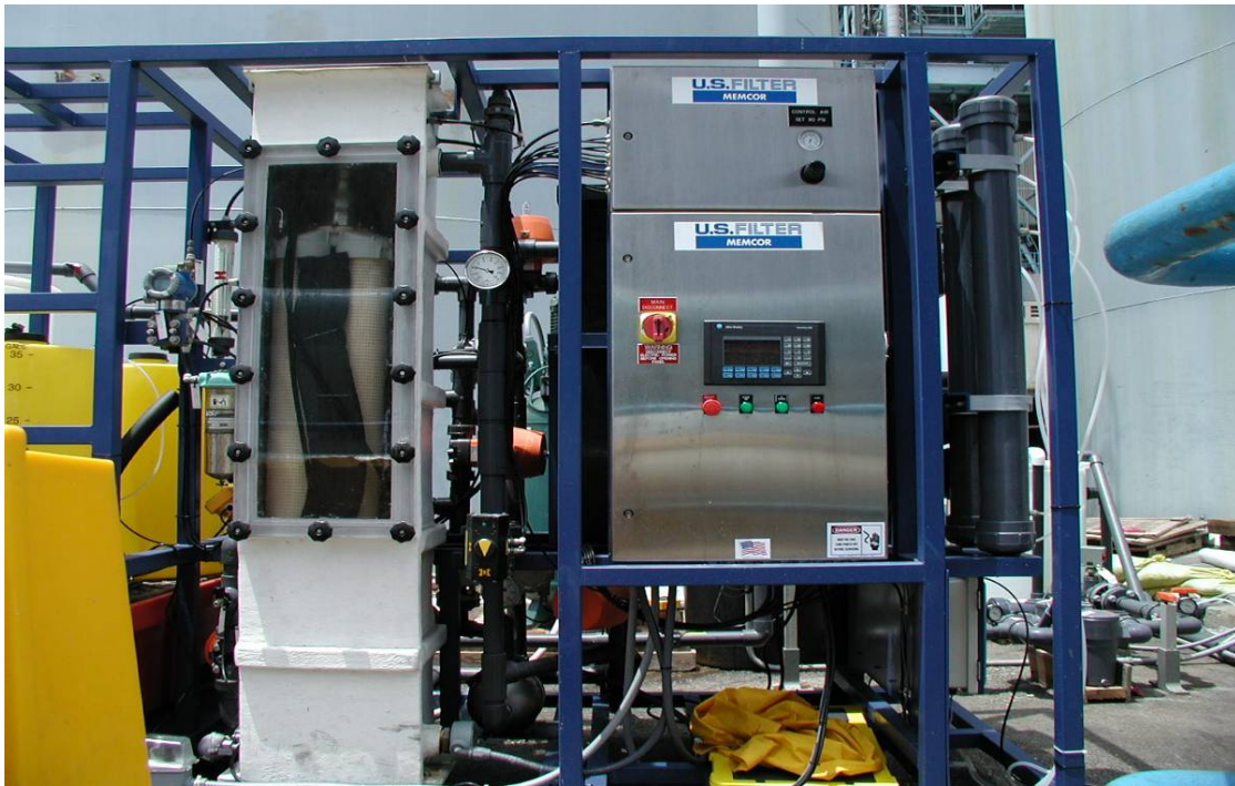
Figure 5.—Siemens CMF-S microfiltration pilot system.
