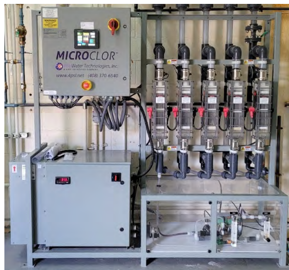
Figure 8 – Chlorine Dosing Equipment
