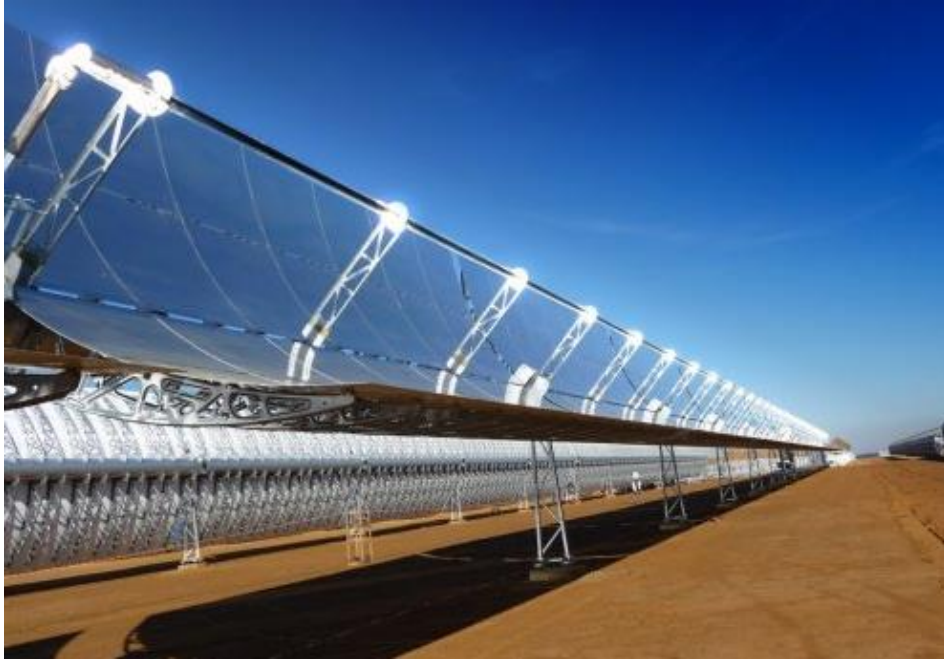
Figure 27: Parabolic through system
