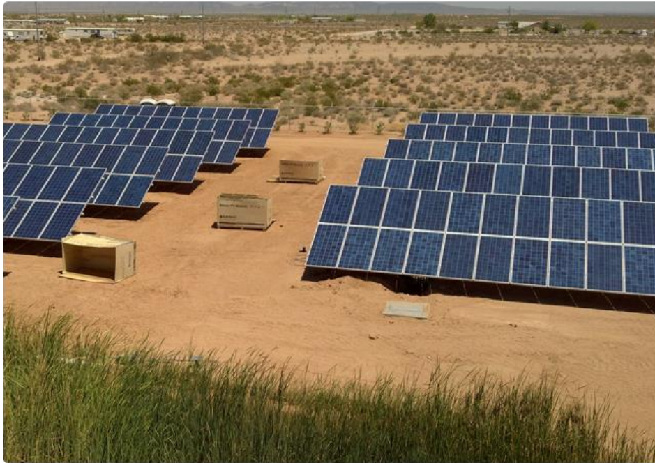
Figure 30: Solar PV plant powering Desalination plant in Yuma, Arizona [50]
