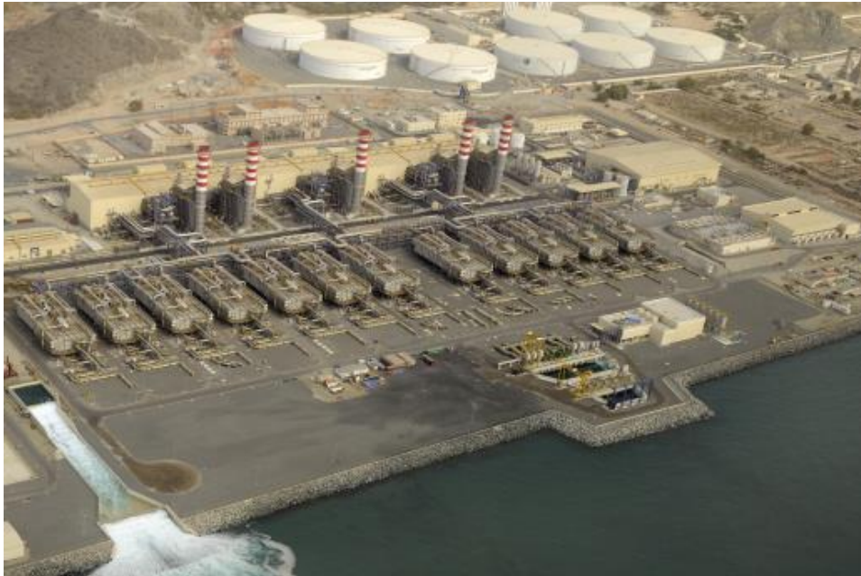
Figure 10: Fujairah F2 MED plant in United Arab Emirates
