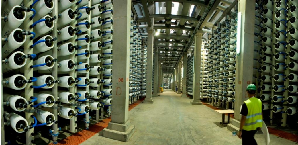
Figure 16: Pressure Vessels at RO Desalination plant in Jordan
