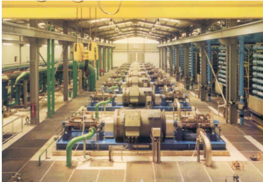
Figure 3.10 Dhekelia Reverse Osmosis Plant 1999
