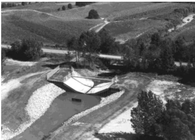
FIGURE 20.5 Goodwin Creek supercritical flow flume (Station #2) that serves as a grade control structure and flow and sediment discharge monitoring station.
