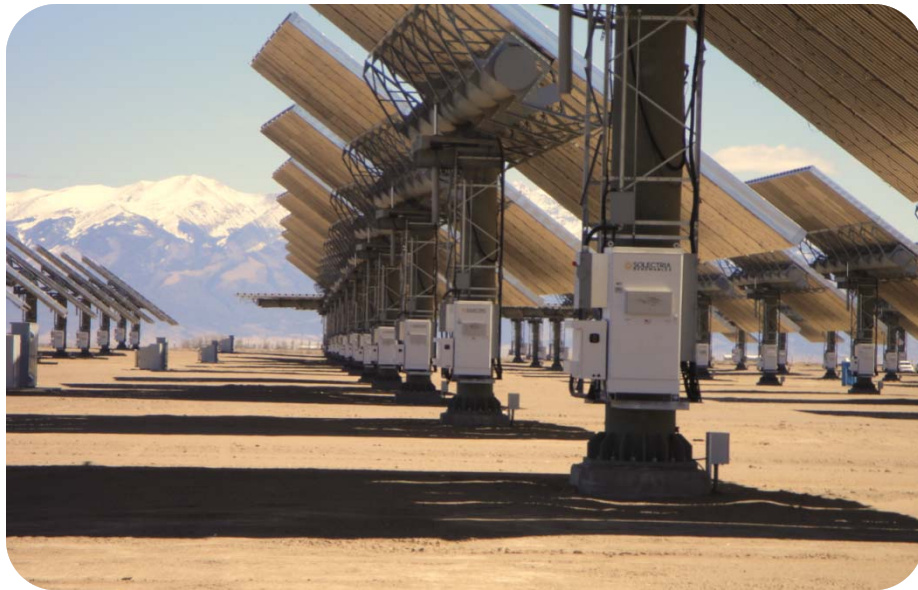
30MW: Qty. 504- PVI 82kW Inverters
