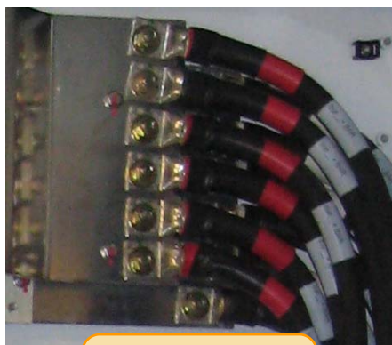
DC bus bar structure
