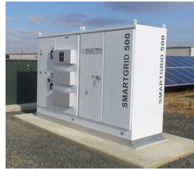
Grid-Tied PV Inverter
