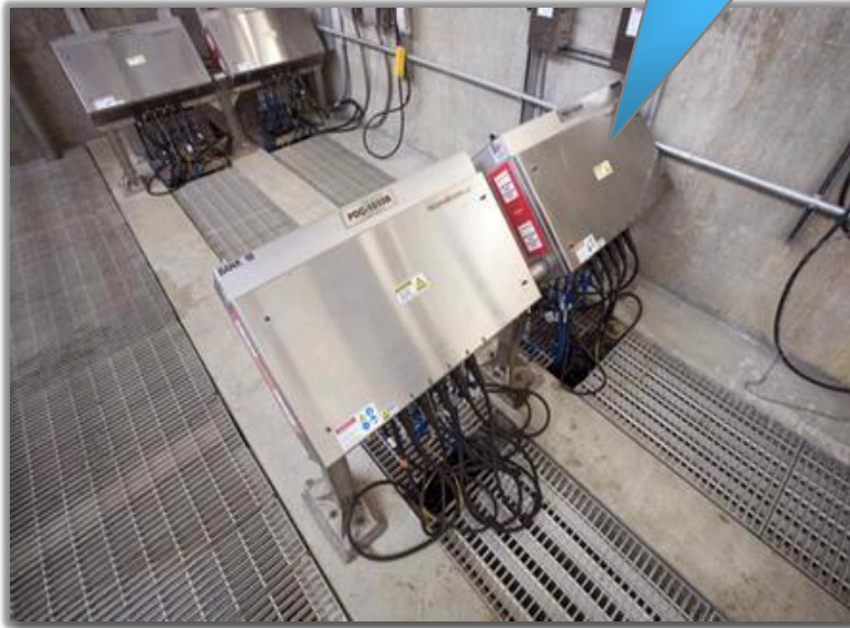
Ultraviolet Disinfection Chamber
