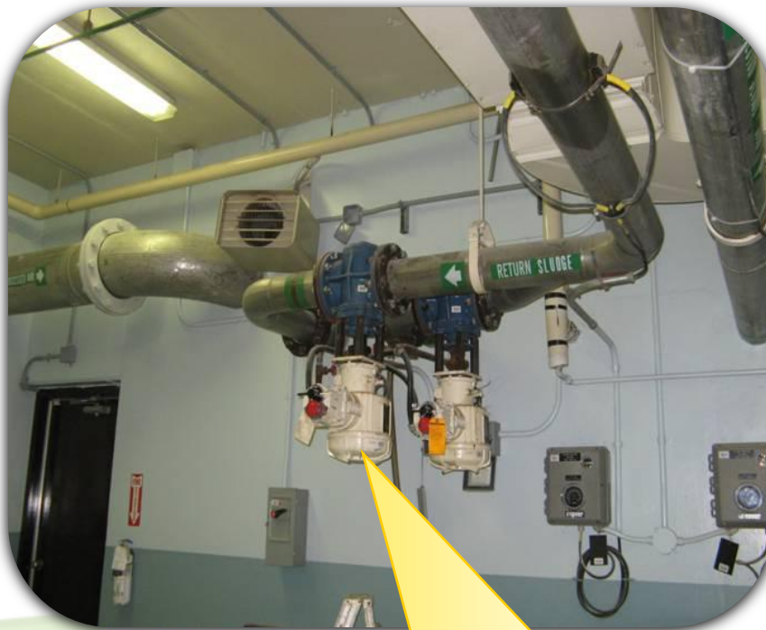
Return Activated Sludge Conveyance System
