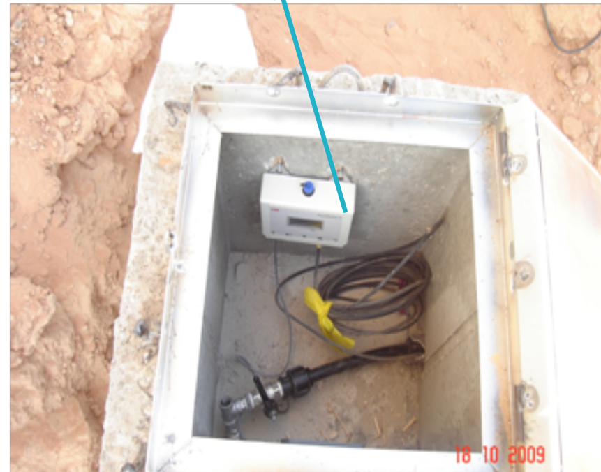
Data loggers in special concrete chambers
