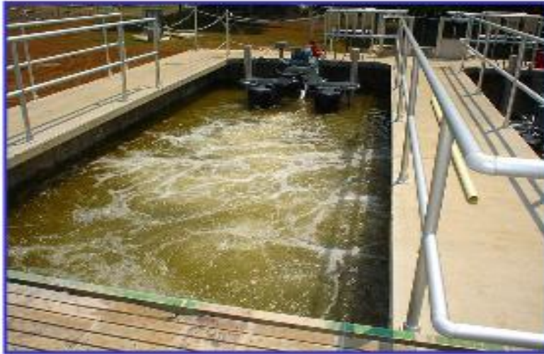
Sequencing Batch Reactors (SBR's)
