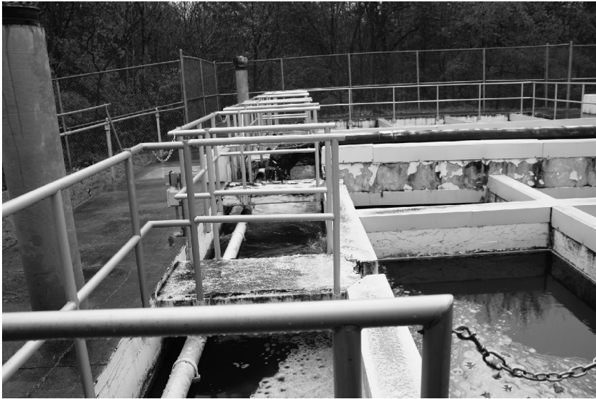
Figure 5.3 Rapid mix basin.
