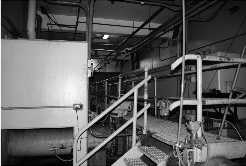
Figure 7.6 Filter backwash and effluent pipes and valves.
