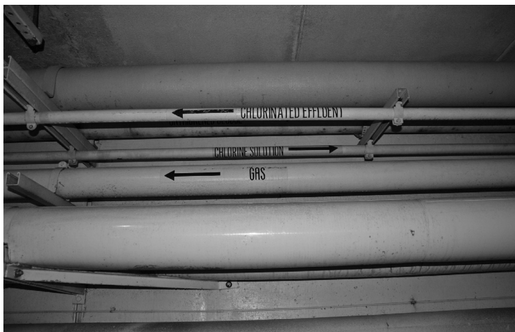
Figure 19.2 Chemical feed lines.
