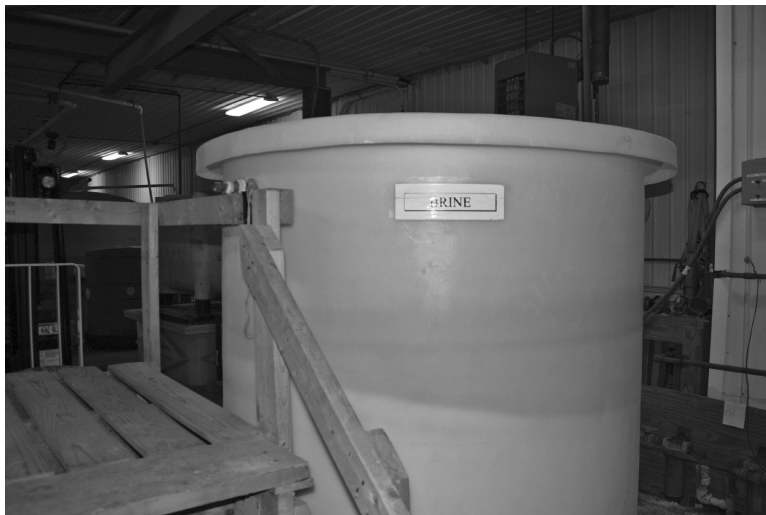
Figure 8.5 Brine for use with mixed-oxidant generator.
