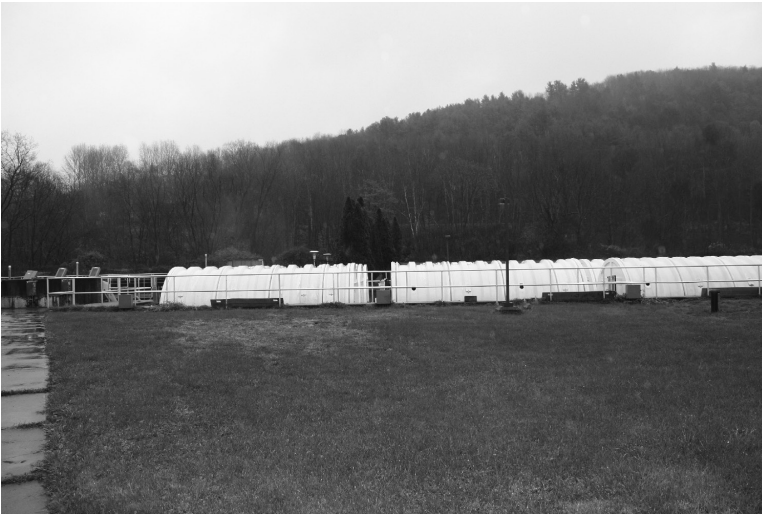
Figure 16.4 Rotating biological contactors.
