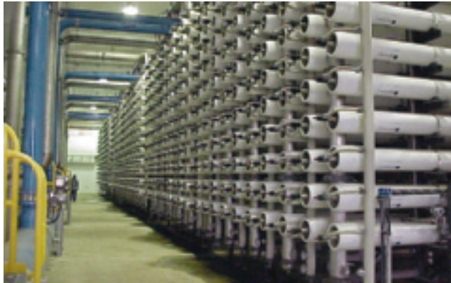
Figure 1.10 Seawater reverse osmosis membrane filtration installation in Larnaka, Cyprus. The permeate production capacity is 54,000m 3 /day. The total amount of eight-inch diameter membrane elements is 5,800. The plant size can be estimated from the person shown on the left of the figure
