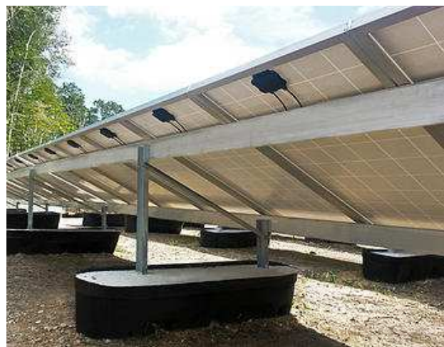
Figure 44: Self-Ballasted Racking Systems Can Avoid Buried Foundation Requirements (Source: GameChange)
