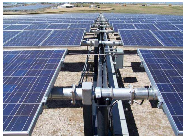
Figure 40: Active Sun-Tracking Arrays Use Hydraulic Pistons or Motors to Drive the Tracking Mechanism for Multiple Subarrays
