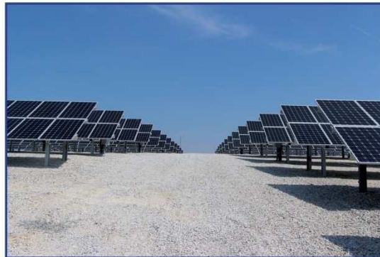
Illinois Rural Electric Cooperative – 500kW
