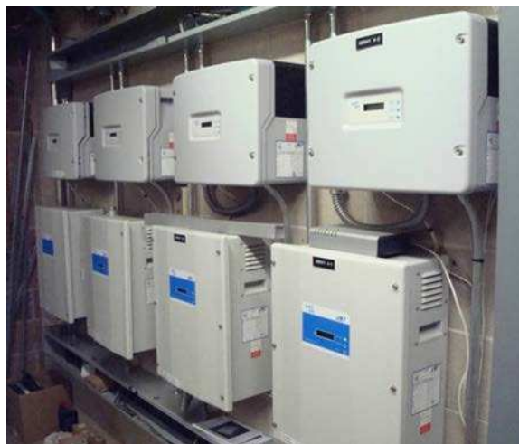
Figure 33: String Inverters Use Series-Connected Array Designs
