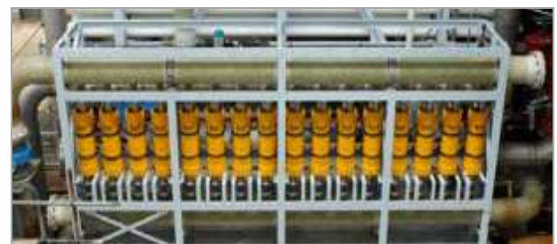
Figure 36: PX device array serving one SWRO train in Perth Desalination Plant (Stove 2008)
