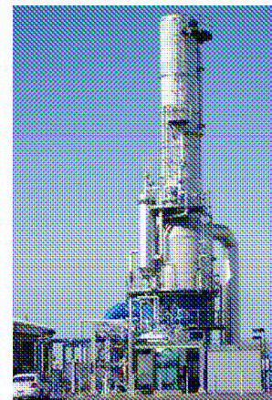
Figure 15: ZLD Water Treatment Facility at D.V.I. in California
