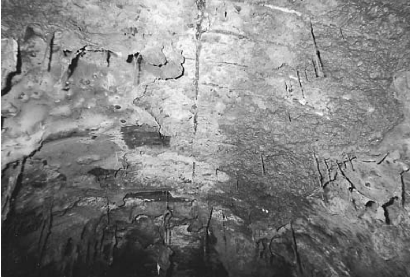
Figure 22.1. Crown corrosion in a sewerage system in Flanders.
