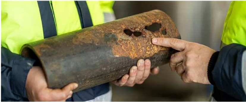
Figure CS8.2 Analysing leak holes in pipe samples.
