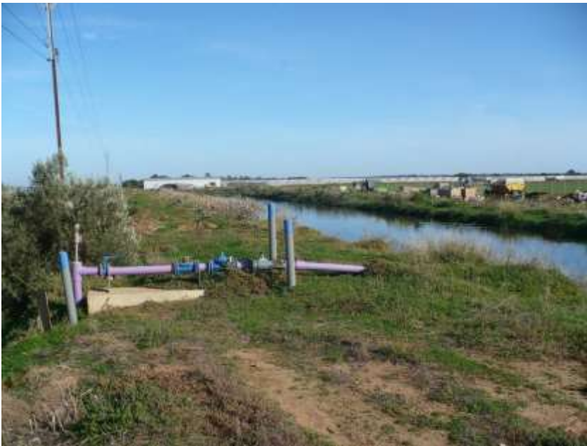
Figure 17.4. Recycled wastewater from the City of Adelaide, Australia is pumped into an irrigation pond for a vegetable farm. Wastewater-conveying pipes are painted purple to distinguish them from fresh water conduits.
