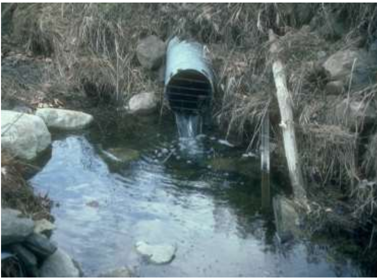
Figure 17.19 Subsurface drain line discharges into an edge-of-field ditch, diverting groundwater to surface waters.
