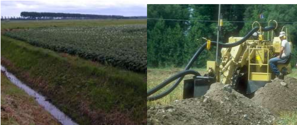
Figure 17.13 Drainage ditch removes excess water and lowers water table (left). Installation of perforated corrugated PVC drain lines using a laser-guided trencher (right).
