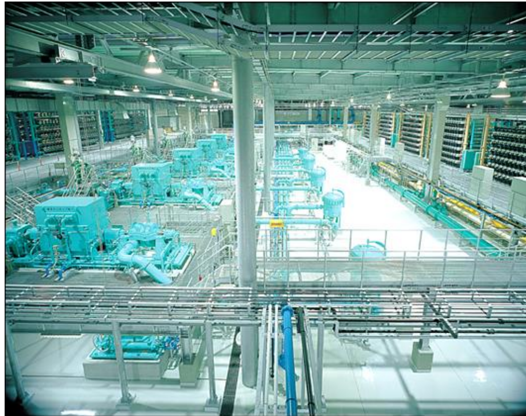
Nata Sea Water Desalination Plant in Japan
