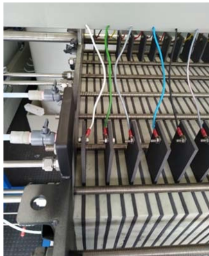
Figure 5.29 Electrical connections of the MDC pilot stack. Source: Author's own work/property.
