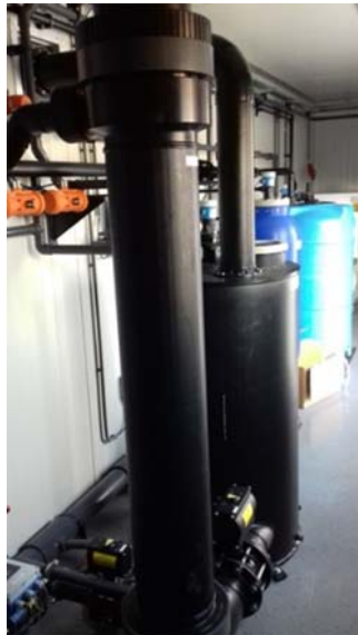
Figure 5.4 Ceramic membranes housed inside a pressure vessel. Source: Author's own work/property.
