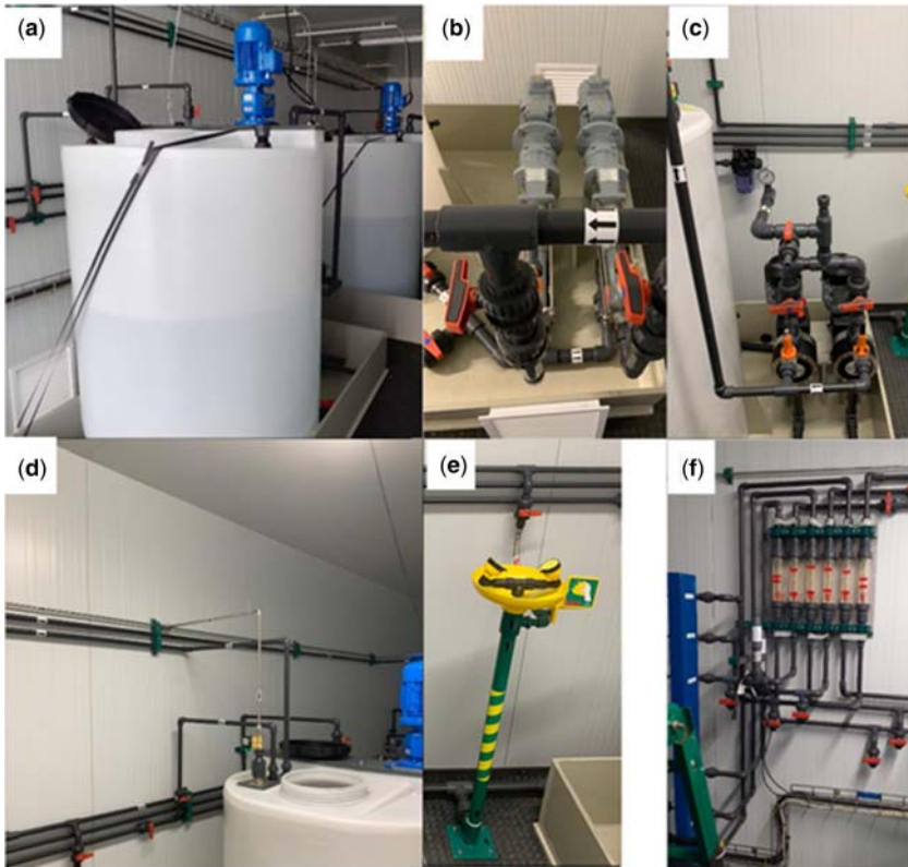
Figure 5.25 Pictures of some of the peripheral elements installed in the MDC pilot plant. (a) tanks, (b) saline and anolyte streams pumps, (c) catholyte stream pumps, (d) pipes and gas line, (e) eyewash and (f) rotameters. Source: Author's own work/property.
