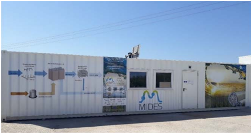
Figure 5.7 Outside view of the ceramic membrane pilot plant container. Source: Author's own work/property.
