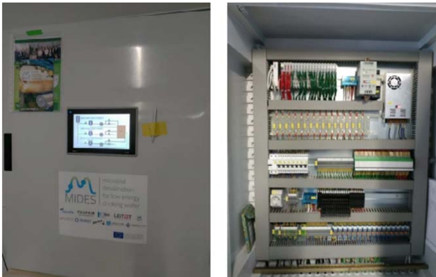
Figure 6.26 MIDES pre-pilot control system switchboard: external and internal views (MIDES Consortium).
