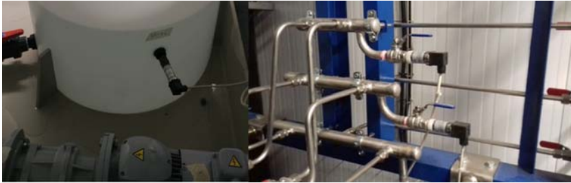
Figure 5.30 Image of the level transmitter located in the tank (left) and pressure transmitters installed in the inlet and outlet of the stack (right). Source: Author's own work/property.
