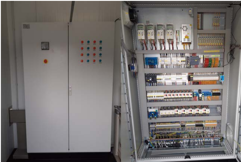
Figure 5.26 Electric panel inside the MDC. Source: Author's own work/property.
