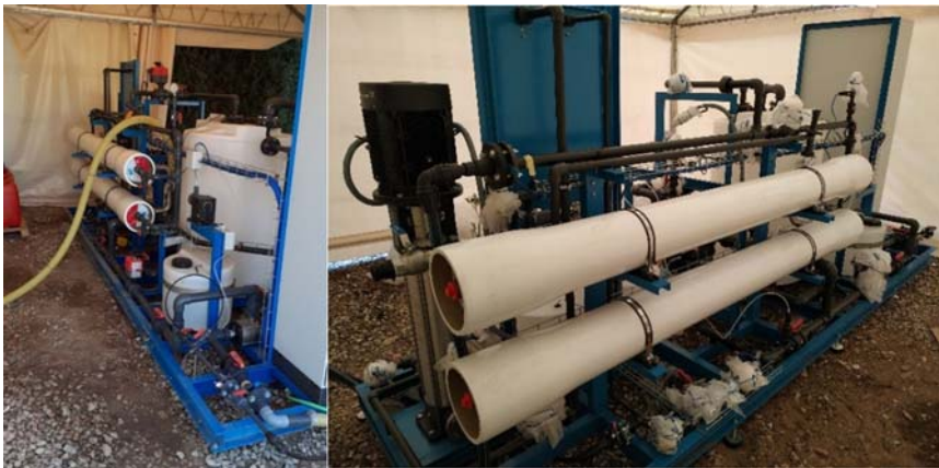
Figure 5.10 RO pilot plant. Source: Author's own work/property.
