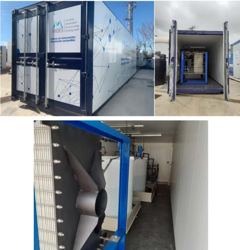
Figure 5.33 Images of the MDC pilot plant located at the Demo Site 1 (Denia). Source: Author's own work/property.
