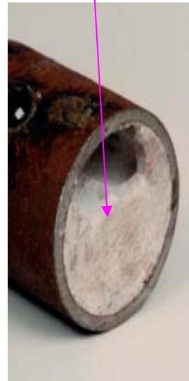
Boiler scale on water side
