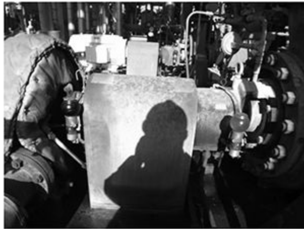
Figure 7.6—Oil bowls on a centrifugal pump with turbine driver
