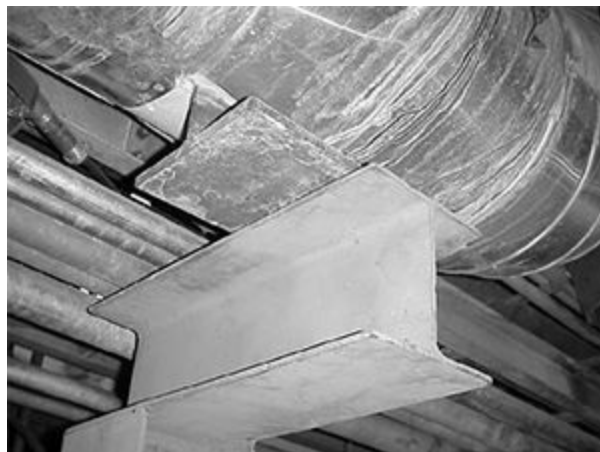
Figure 7.15—Pipe shoe not contacting pipe support
