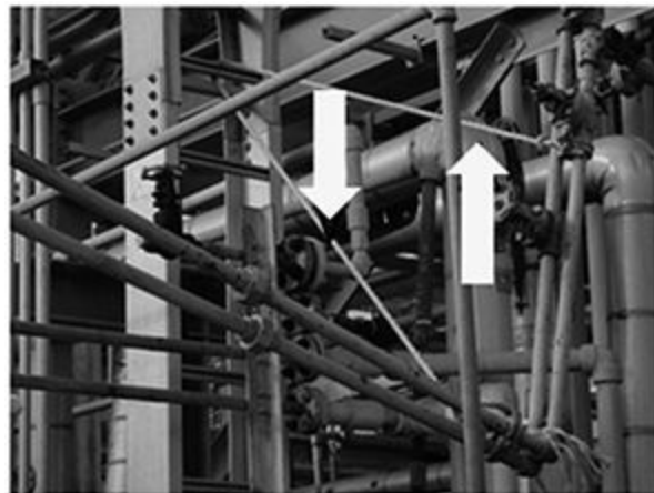
Figure 7.4—A rope support has slipped and cocked the pipe
