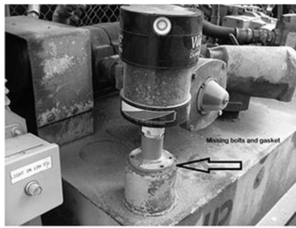
Figure 6.1 Desiccant appears to have reached half its useful life. Notice, the missing attachment bolts and gasket.
