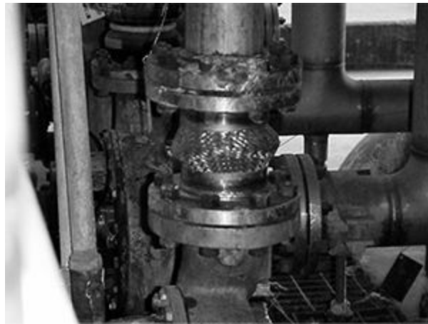
Figure 7.9—Over-compressed expansion joint
