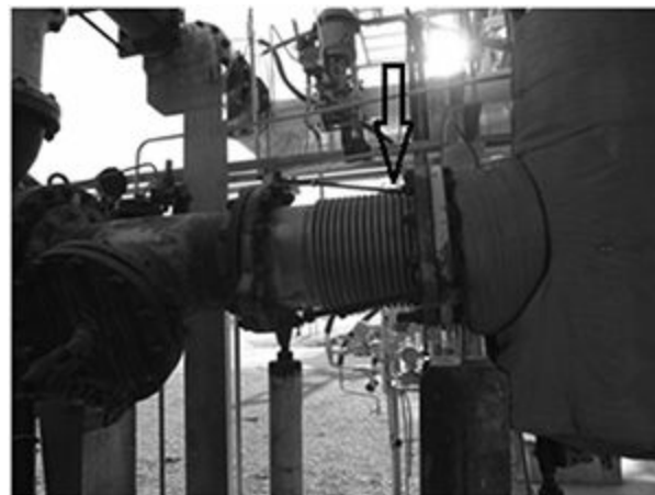
Figure 7.10 Expansion joint loose stay rods
