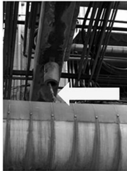
Figure 7.3—Hanger support is broken
