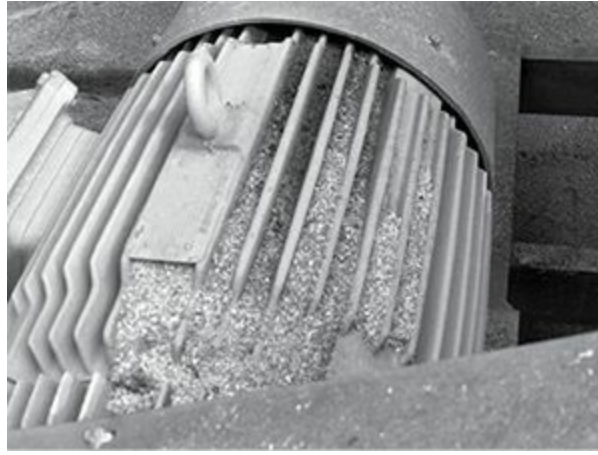
Figure 4.4—A TEFC (totally enclosed fan cooled) electric motor with debris resting between the cooling fins. This reduces the motor's ability to expel internal heat, which could lead to overheating and the eventual failure of the internal windings.
