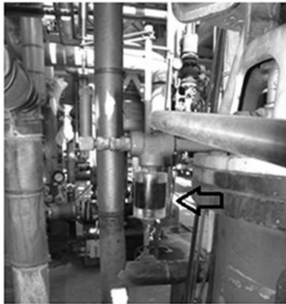
Figure 7.14—Oil sight on sump
