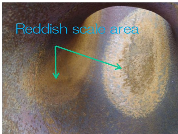
Color changed area of inside piping
