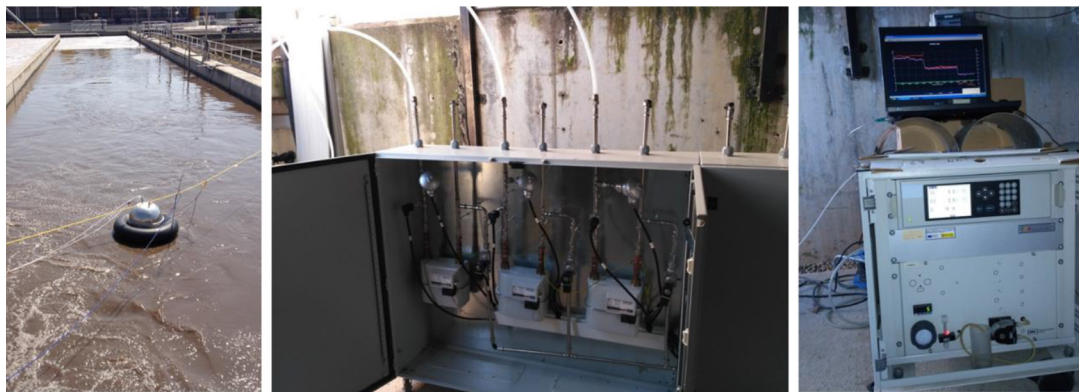
Figure 5.7 Floating hood (configurations C and E in Figure 5.6) and associated equipment for measuring off-gas flowrates and off-gas concentrations. Photos courtesy of Dr. Maite Pijuan (ICRA Catalan Institute for Water Research). These figures were published in Journal of Cleaner Production , Vol number 212, A. Ribera-Guardia, L. Bosch, L. Corominas, M. Pijuan, Nitrous oxide and methane emissions from a plug-flow full-scale bioreactor and assessment of its carbon footprint, Page Nos 162–172, Copyright Elsevier (2019) and in Science of the Total Environment , Vol number 493, A. Rodriguez-Caballero, I. Aymericha, M. Poch, M. Pijuan, Evaluation of process conditions triggering emissions of green-house gases from a biological wastewater treatment system, Page Nos 348–391, Copyright Elsevier (2014).
