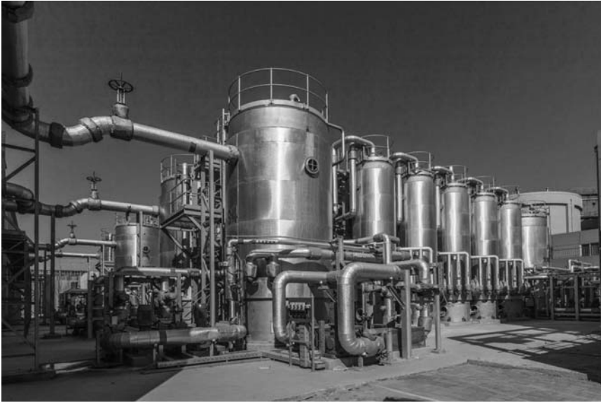
Figure 6.9 Thermal hydrolysis installation in Gaobeidian, Beijing. Photo courtesy of Cambi.
