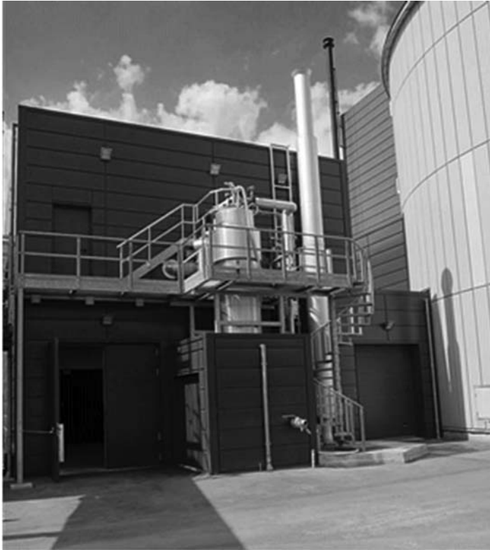
Figure 6.7 Thermal hydrolysis unit at Billund Biorefinery. (Courtesy: S. Viswanathan).
