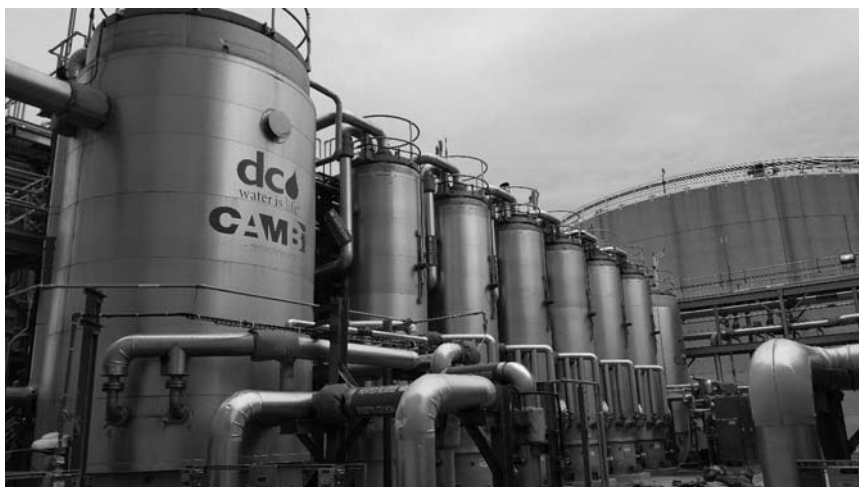
Figure 6.5 Photo of the thermal hydrolysis plant in DC Water (Photo by author).
