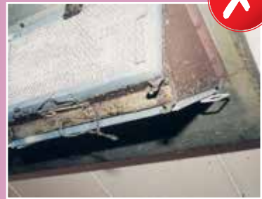
Cleaning schedules should prevent dirt and dust build-up and other cleaning problems
