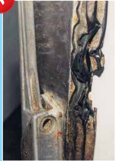
Defective refrigerator door seals should be replaced
