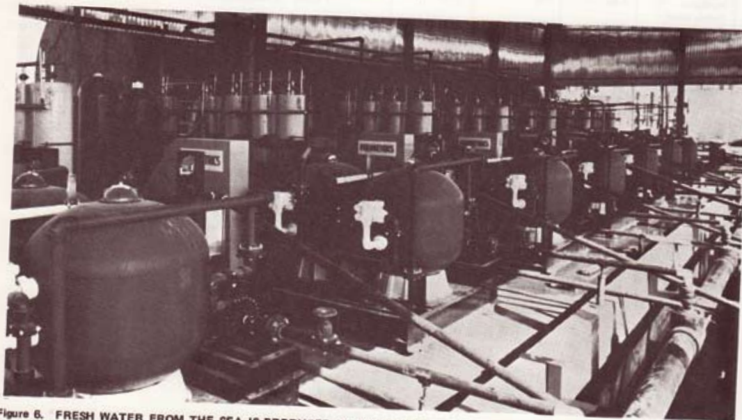
Figure 6. FRESH WATER FROM THE SEA IS PRODUCED IN RAS AL KHAIMAH, UNITED ARAB EMIRATES, BY THIS 150,000-GALLON-PER-DAY DESALTING FACILITY USING 8-INCH DIAMETER Du PONT REVERSE OSMOSIS 8-10 "PERMASEP" PERMEATORS. THE FRESH WATER IS USED BY AN ADJACENT CONCRETE PLANT WHICH MAKES PRECAST CONCRETE FOR USE IN NEARBY SAUDI ARABIA.
