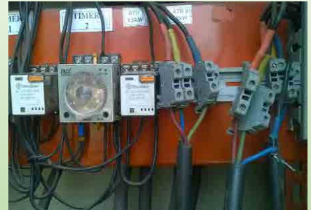
Exposed electrical parts
