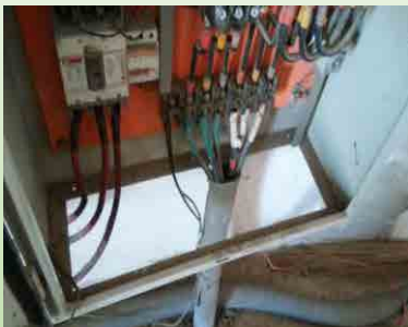
Broken base plate
