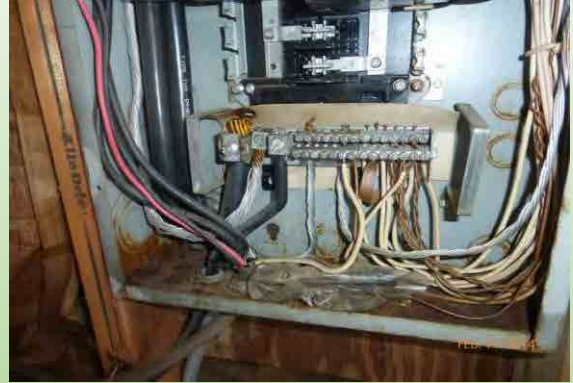
Wet & moist condition
