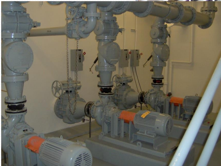
Raw Sewage Pumps
