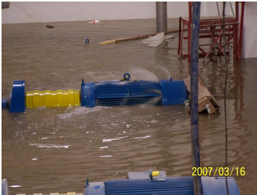
Dry Pit Pump Basement
