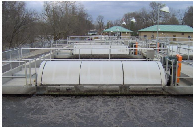
Vertical Loop Reactor
