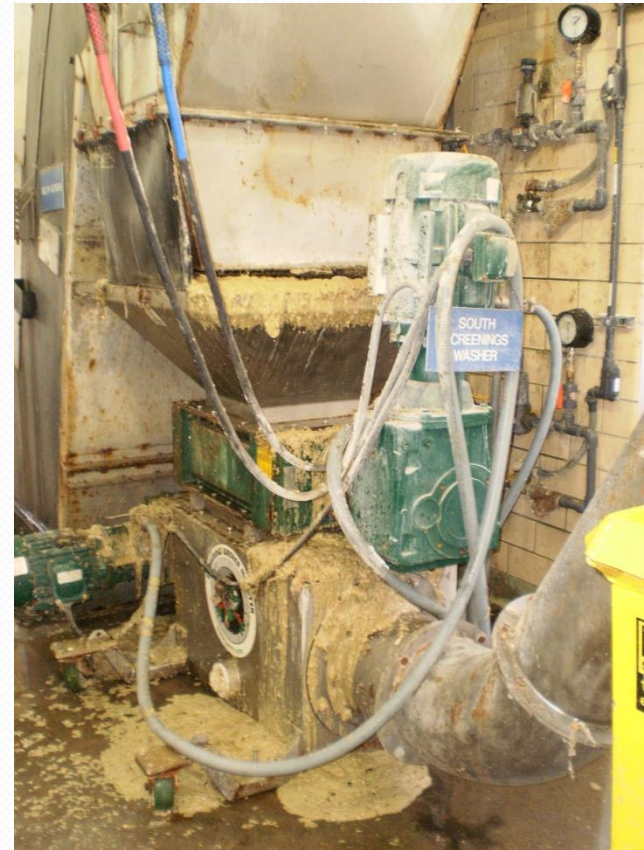
Excessive Grease in Bar Screen
