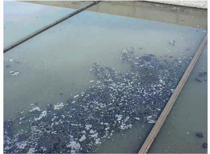
Rising septic sludge in primary clarifier
