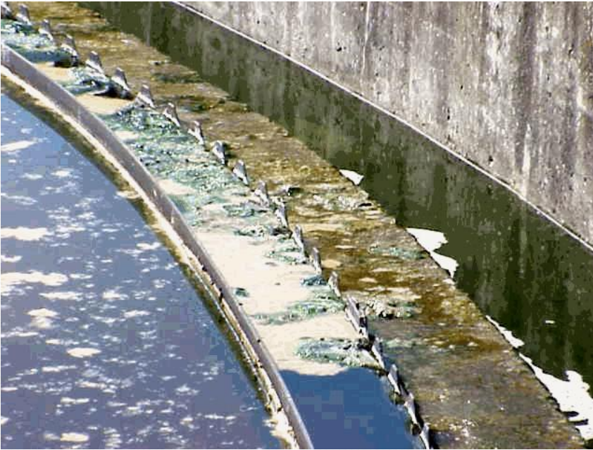
Scum blocking weirs causing short circuiting
