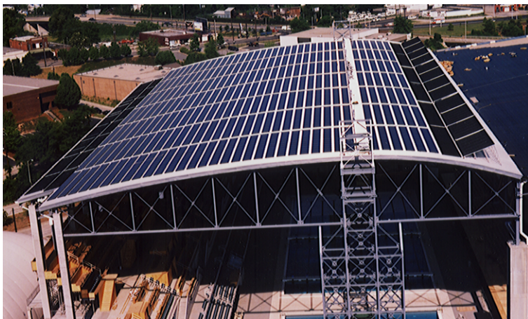
Figure 8.2 Roof-mounted PV ( Source: U.S. National Renewable Energy Laboratory ).
