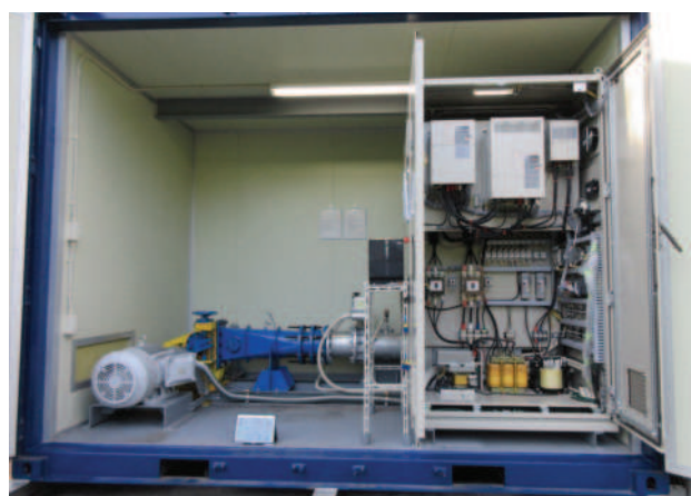
Figure 3. Equipment of the power plant
