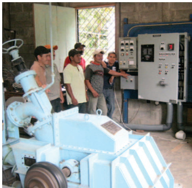
Figure 7. ATDER-BL technical team in the Bocay powerhouse
