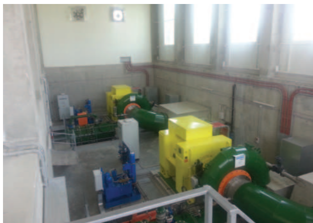
Figure 2. Inside Akhmeta SHP
