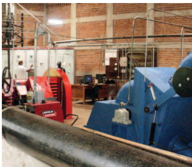
Figure 4. Equipment in EL Bote powerhouse
