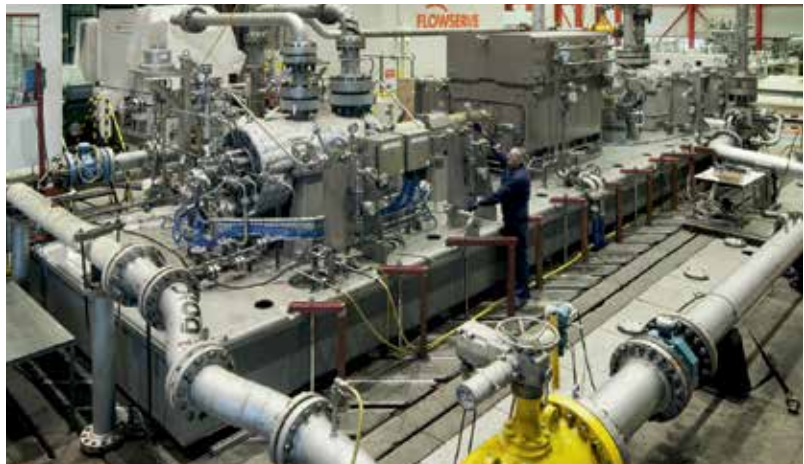
Typical power recovery train unit
