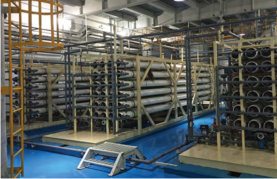
Figure 5: Power Plant MBC System
