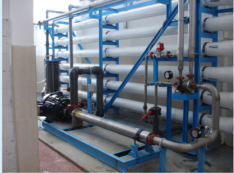
Photo 3 —Small Turbocharger on RO Skid
