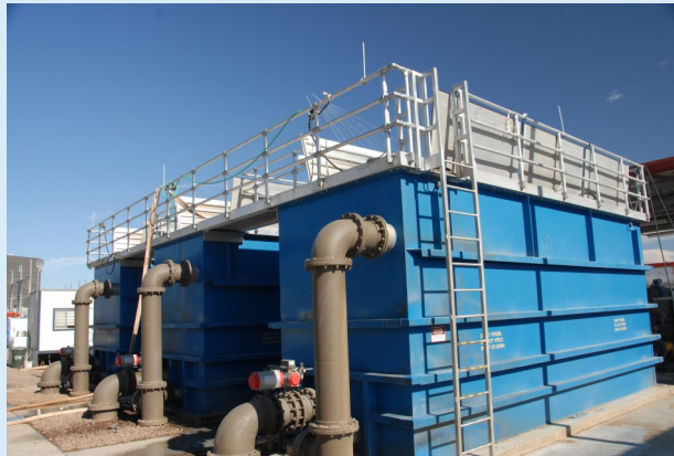
This food processing facility uses MBR and RO to recover process water and minimize the water footprint at a highly water stressed location in Arizona.
