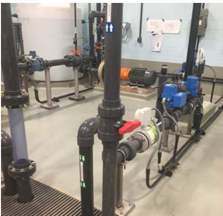
Photo shows a fully automated neutralization system
