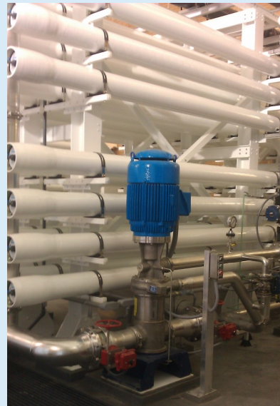
Photo 5 —Motorized Turbocharger on RO Skid
