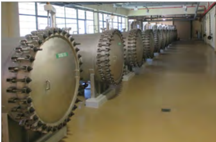
Figure 3: Cartridge Filter Housings for Pretreatment
