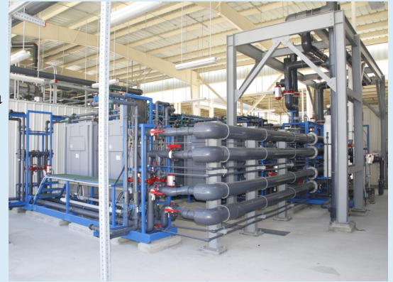
This non-potable reuse facility in California employs Electrodialysis Reversal for the reduction of dissolved solids, supplying a new source of water for irrigation and industrial uses.
