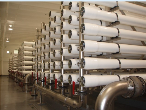
Reverse Osmosis and Nanofiltration trains generate permeate and concentrate
