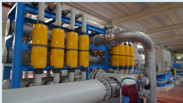
Photo 6 —Pressure Exchange Skid
