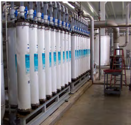
Figure 2: Example of skid mounted UF modules
