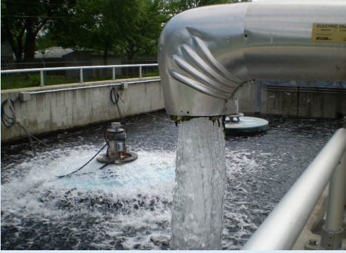
Discharge of concentrate to a mixing tank
