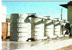
Odor Control at the Master Pumping Station - City of Treasure Island, FL.
