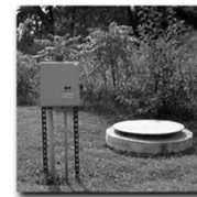
Submersible lift stations are designed to blend readily with natural surroundings, since there is no pump house and there is a minimum of above-ground equipment. Other advantages to below-ground installations are noise reductions and less safety-hazard concerns.
