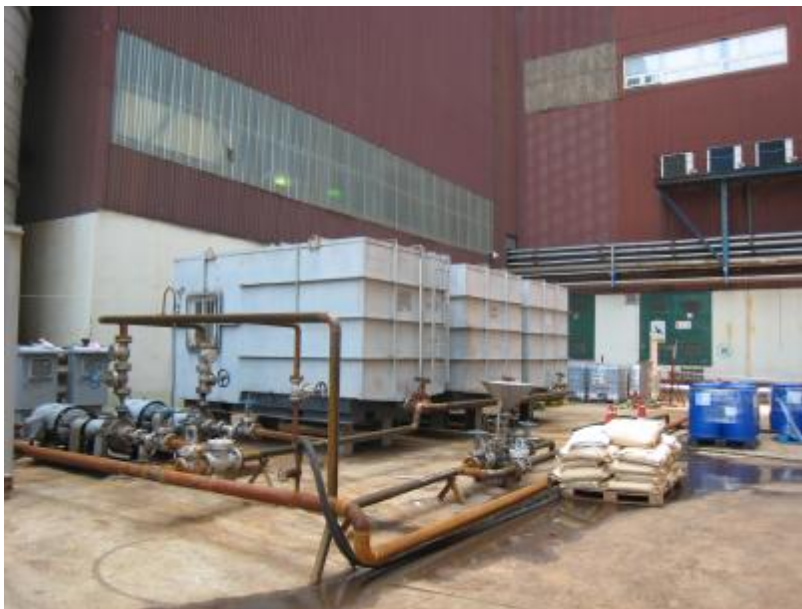
chemicals injection equipment
