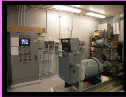
The Main Avenue Pump Station
