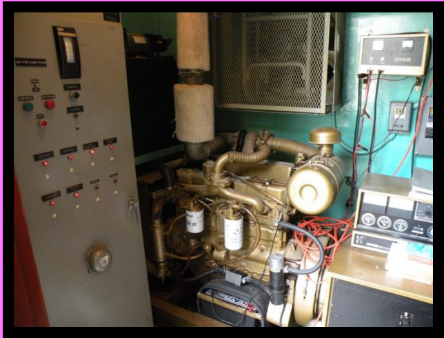
The South Gardiner Pump Station
