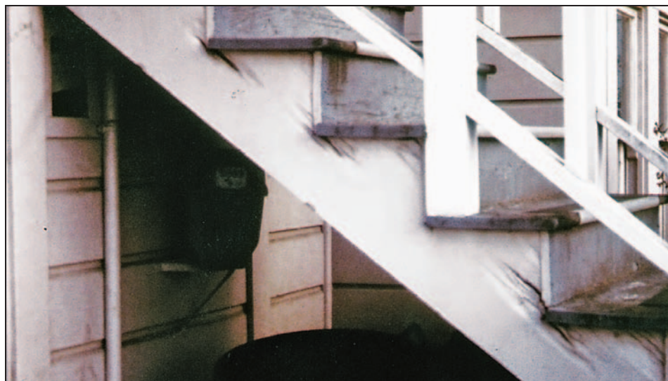
Figure 13-13. Deterioration in a notched stair stringer
