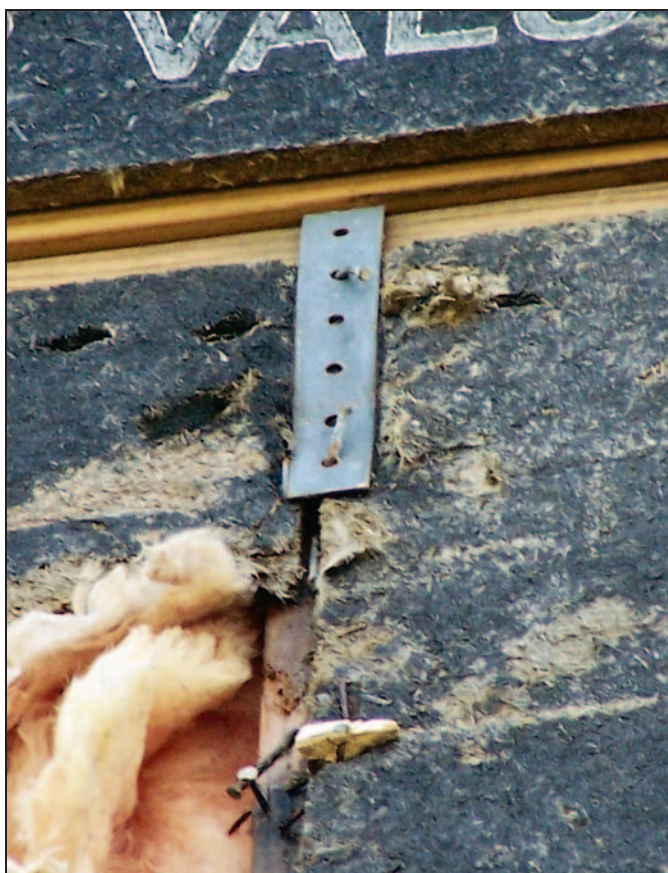
Figure 13-15. Connector failure caused by insufficient nailing
