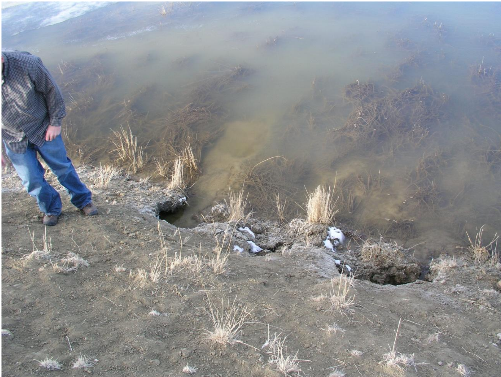
Picture 4 - Sloughed Material
