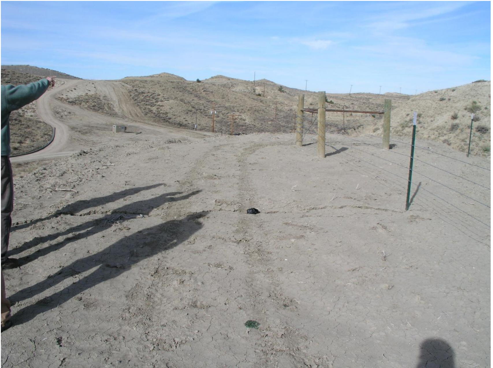
Picture 1 - Horizontal Cracks
